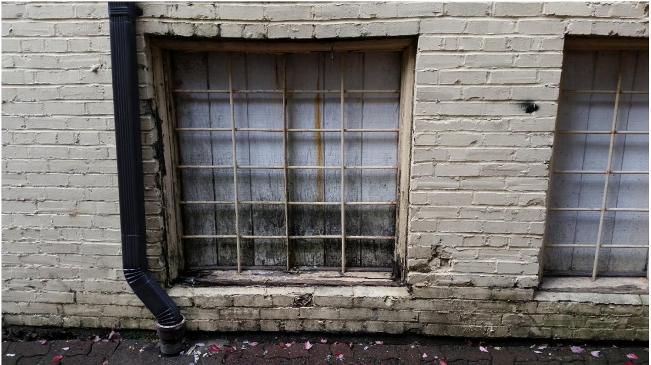
ALLEY WINDOW SHOWING BOW OF THE BRICK AND THE CONDITION OF THE WINDOWS
