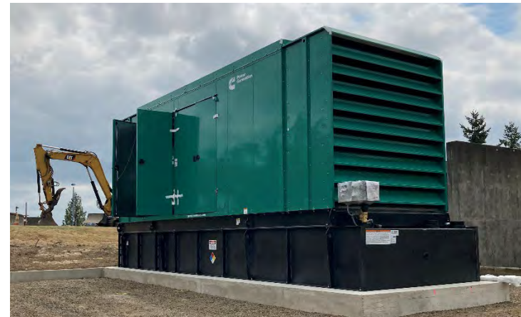
The City continued to invest in upgrades to the public sanitary sewer system in 2021. Work included installation of 1000 KW generators at the Water Reclamation Facility and the Raw Sewage Pump Station.
