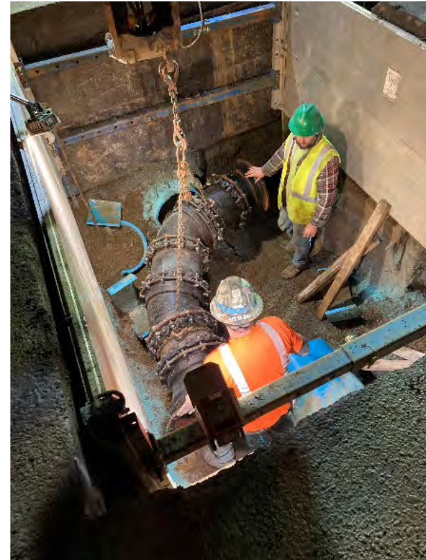
Installation of the temporary sanitary sewer force main Three Mile Lane bridge crossing to allow construction of the new bridge.
