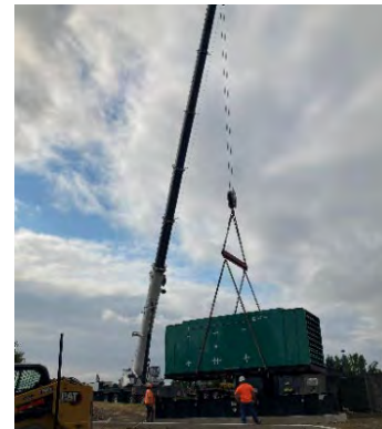
To provide actual redundant power, two generators were installed. One at the Water Reclamation Facility, and the other at the Raw Sewage Pump Station (RSPS).
