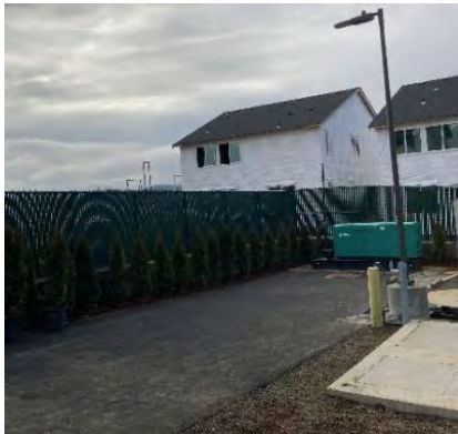
A new pump station was added at the corner of NW Charles St and NW Alfred Dr to service the new development in the area.
