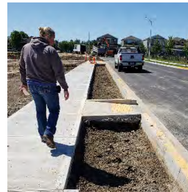
Park Maintenance Supervisor Liz Fliszar (14 years) performs construction inspection at Jay Pearson Park
