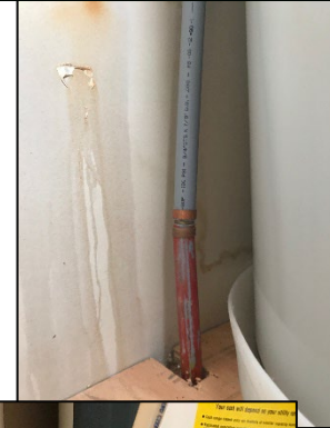
Leaking Grey Pipe
