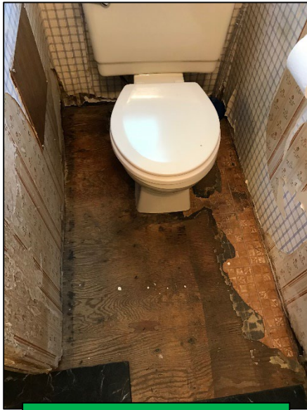
Leaking Toilet & Water Damage
