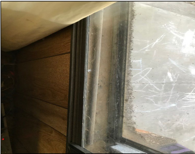
Seeping Windows. Dry Rot & Mildew Throughout.
