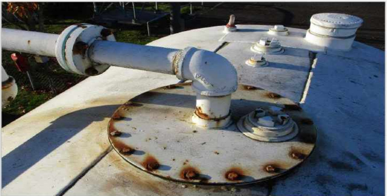
Exhibit "A" Paint failure and rust on Tank
