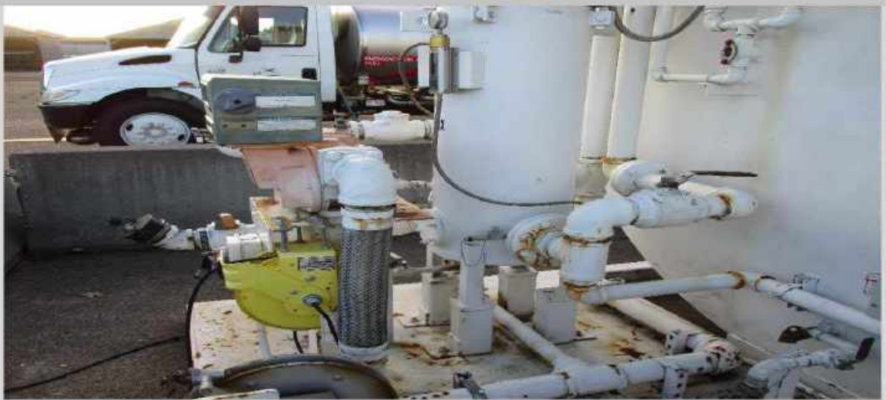
Exhibit "A" Paint failure and Rust on tank
