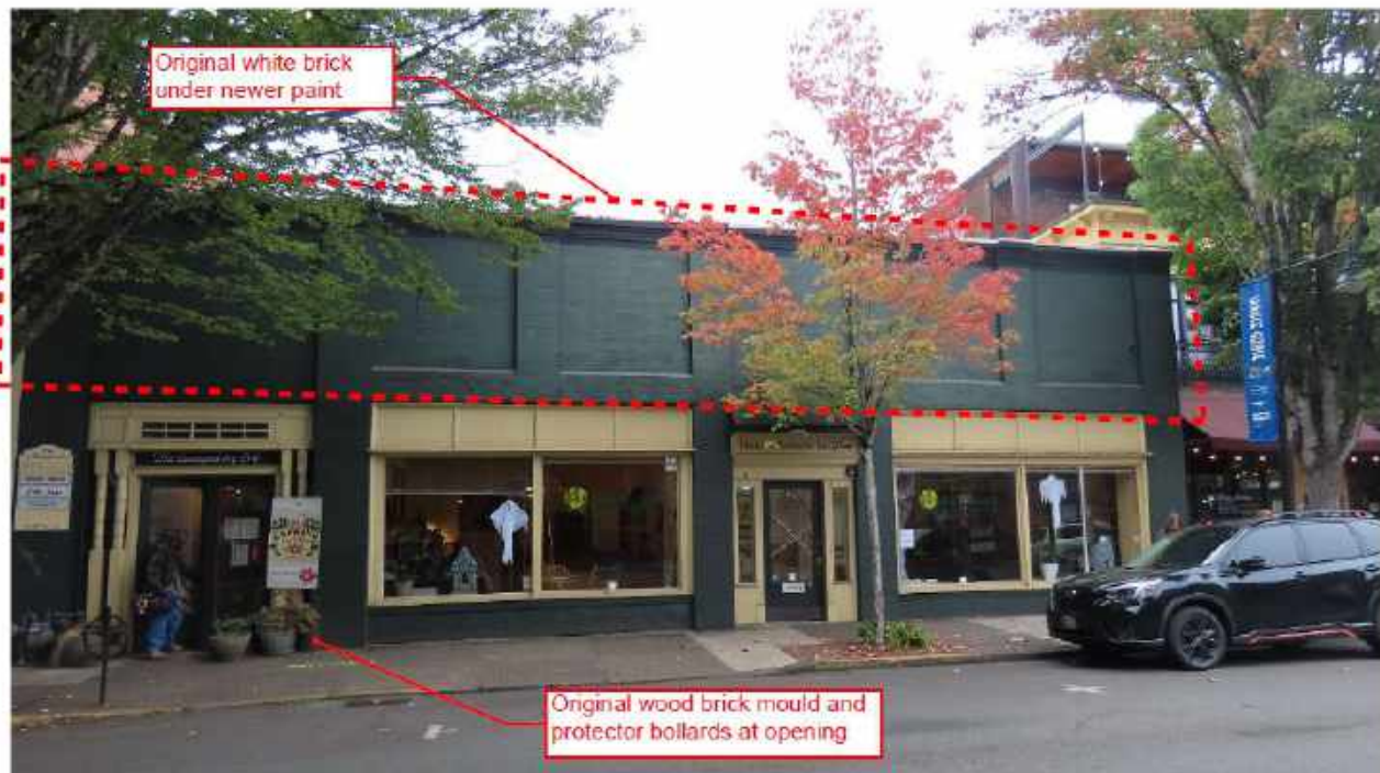
Current view of 619 NE 3rd Street (ARG, October 2022). Paired doors with wood trim elements have been inserted into the westernmost bay, while the formerly double-wide opening has been replaced with a storefront window matching the window in the easternmost bays.
