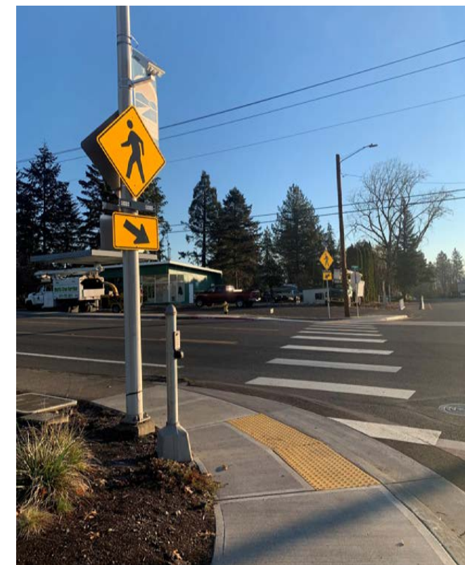
Rectangular Rapid Flashing Beacon
