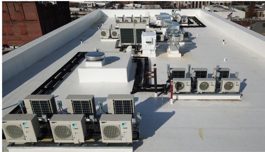
Atticus Hotel rooftop equipment, roof approx. 6,600 SF
