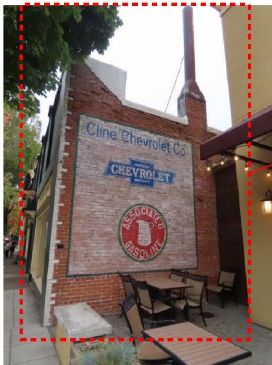
619 NE 3rd Street, Southwest corner, showing restored signage at east elevation (ARG, October 2022).
