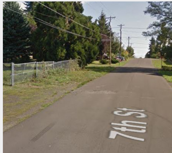
7th St is an important travel route for students who live west of the school. However, there is not a complete walking path for students because of sidewalk gaps between Bridge St and Jefferson St.
