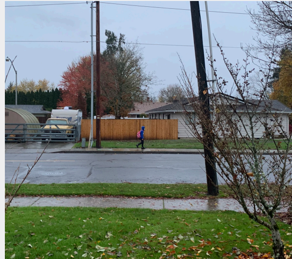
Sidewalks along the east side of Davis St are inconsistent. Some sidewalks near the school were observed to be partially overgrown by vegetation.
