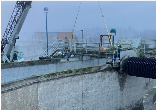
Wastewater Services mechanics guide a shaft as a crane lowers it into place on the oxidation ditch.
