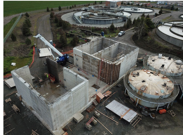
The City continues to invest in upgrades to the public sanitary sewer system in 2024-25 by addressing solids capacity issues with upgrades to our solids handling processes.
