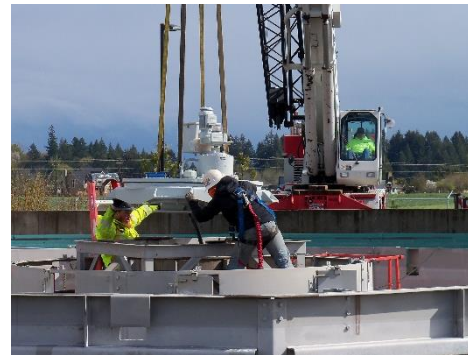
A crew from Stettler Construction uses a crane to install a drive assembly into secondary clarifier #3.
