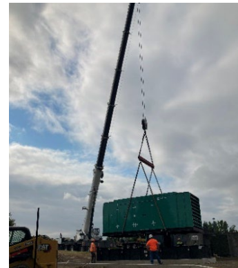
The final generator needed to complete our redundant power requirements at our pump stations will be installed this year at our Cozine Pump Station.
