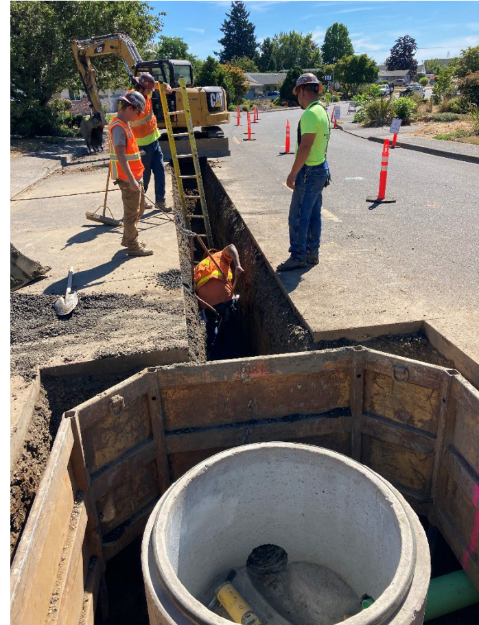
Construction crews work on the NE High School Basin Sanitary Sewer Rehabilitation Project in 2022.
