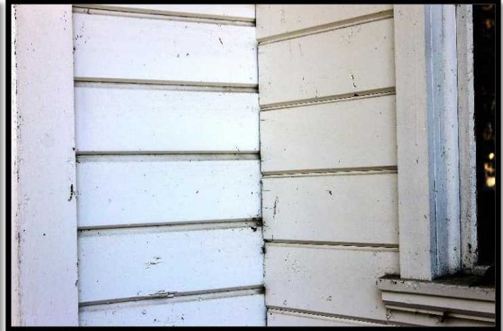
Figure 6: View of external junction between main structure wall and porch addition. Note offset of siding pattern
