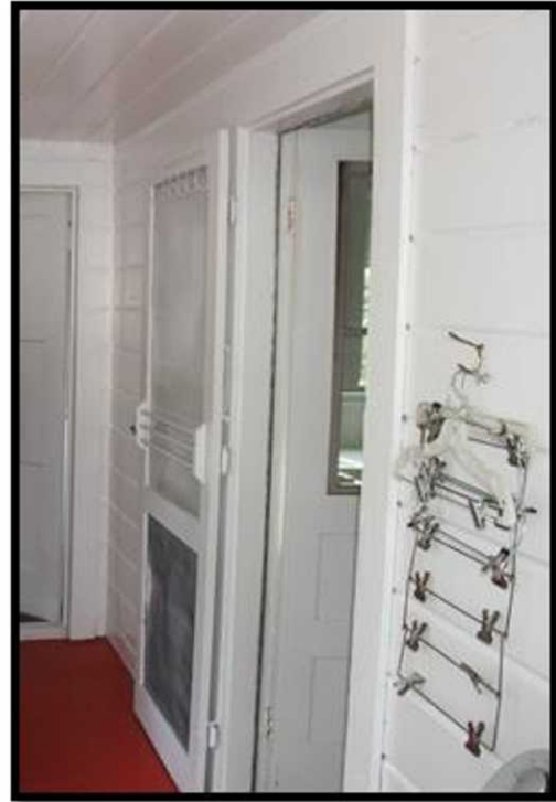
Figure 3: Screen door still in place within interior
