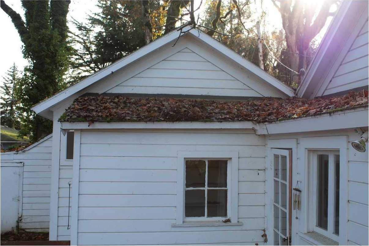
Figure 13: View from North of existing porch structures and roof line. Note also existing window trim.
