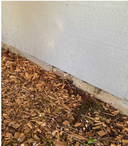
Image 9 College 423 Foundation failure in several spots providing access to vermin.
