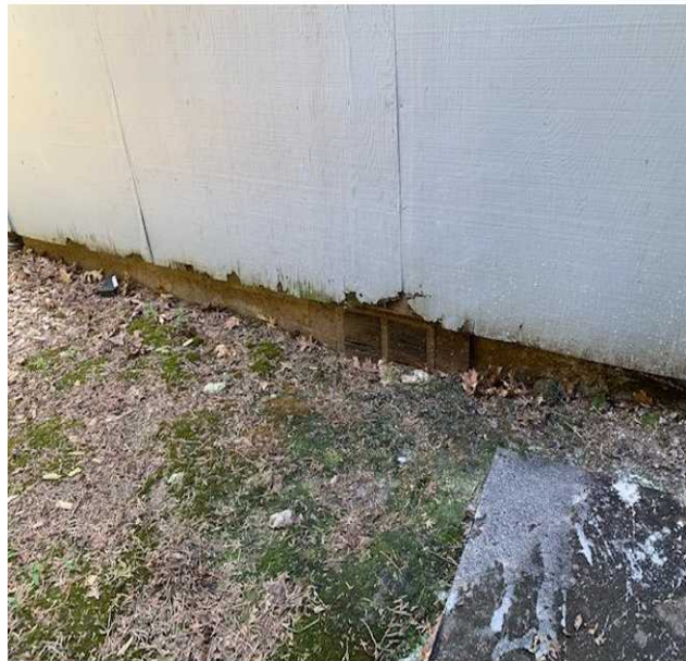
Image 7 College 415 Siding dry rot.
