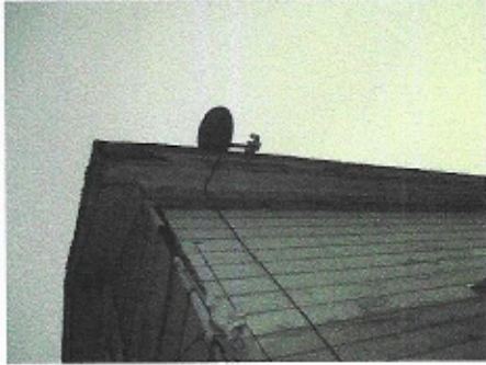
Extensive dry rot, no gutters
