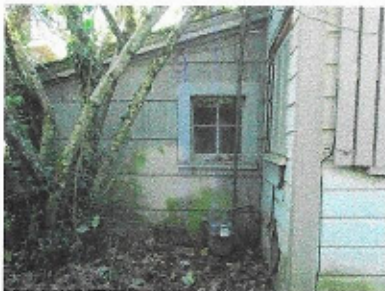
No foundation frame has extensive dry rot due to moisture damage
