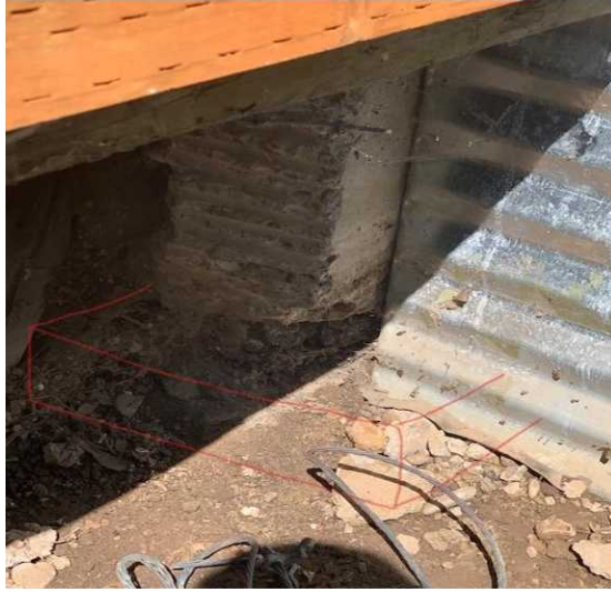
Image 8 College 423 No foundation footing (Similar to College 415)
