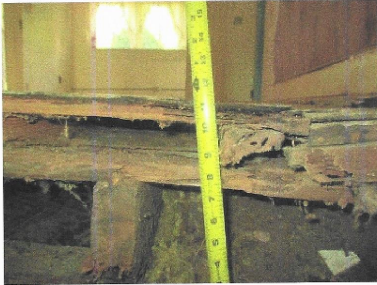
Kitchen extensive dry rot
