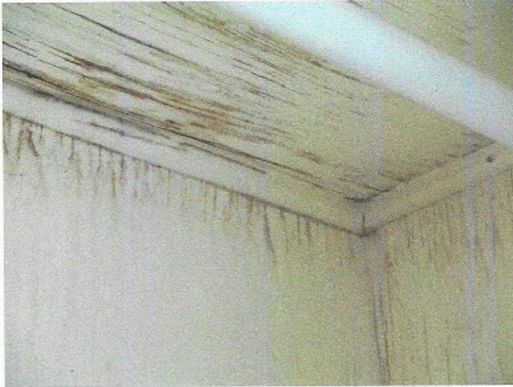
Interior extensive water damage, dry rot.
