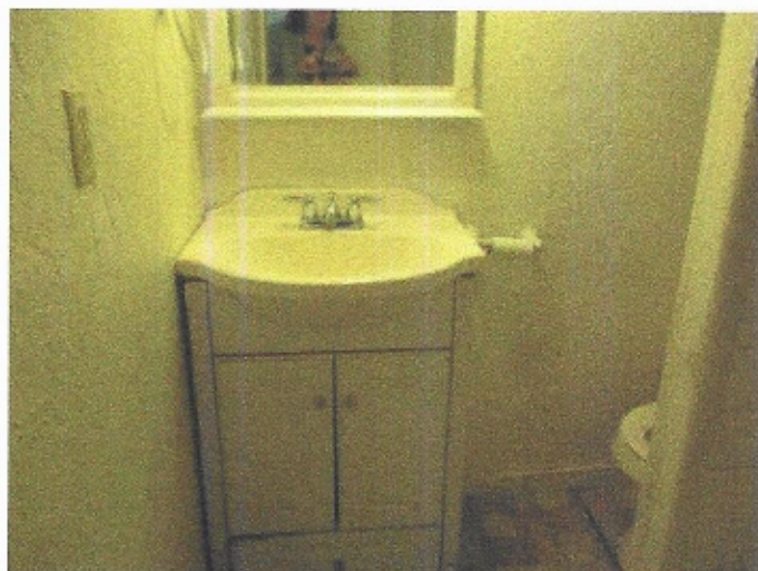
Not original, extensive dry rot and water damage
