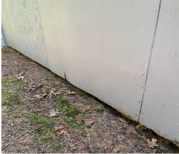
Image 6 College 415 Siding and sole plate dry rot.
