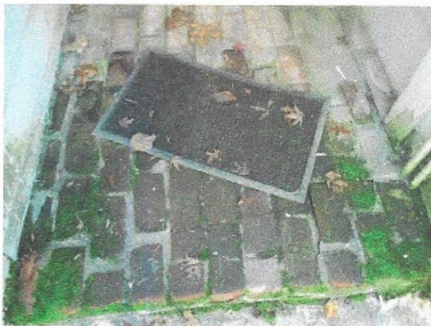
Entrance Brick has sunk about two inches due to dry rot under house due to no moisture barrier and no foundation only sitting eleven inches off the ground.
