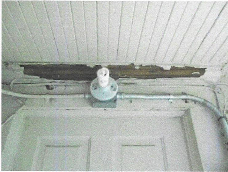
Electrical not up to code
