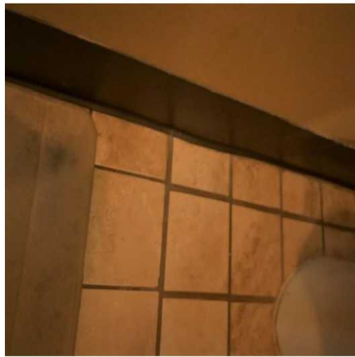
Image 11 College 423 Dry rot floor structure with floor caving in.
