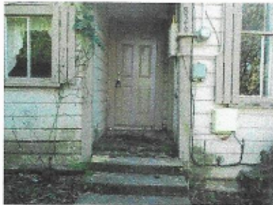
Front entry extensive dry rot
