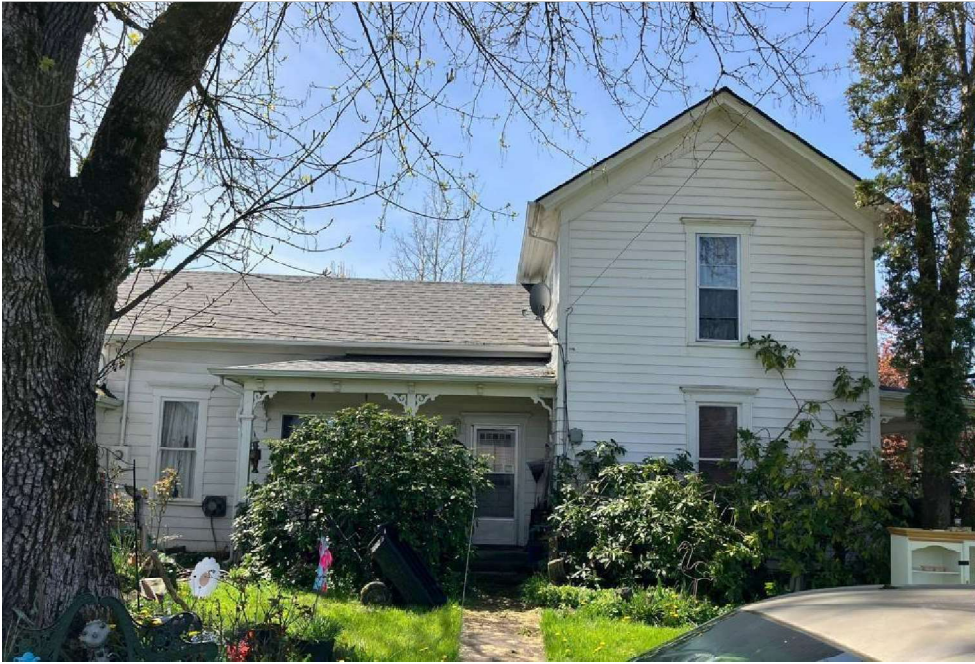
View looking South from Vine St. Siding and most windows appear to be original. Detail on porch is original. Behind large shrub on porch is a double metal window replaced in the late 70s. There is also a wall AC unit installed under the window.
