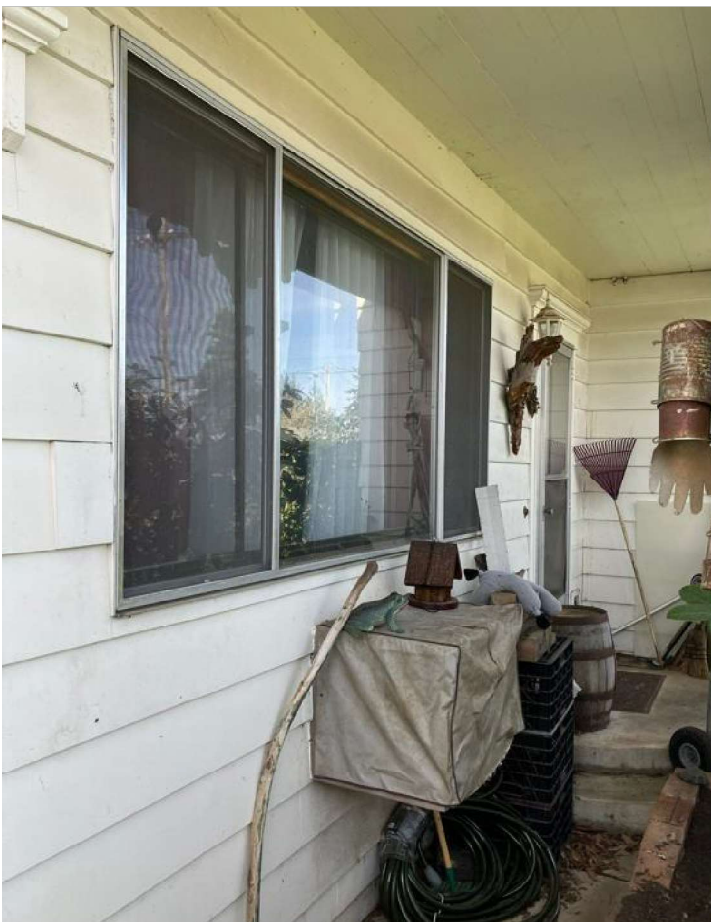
Close up view of porch from photo above. Shows double metal window and wall installed AC unit.
