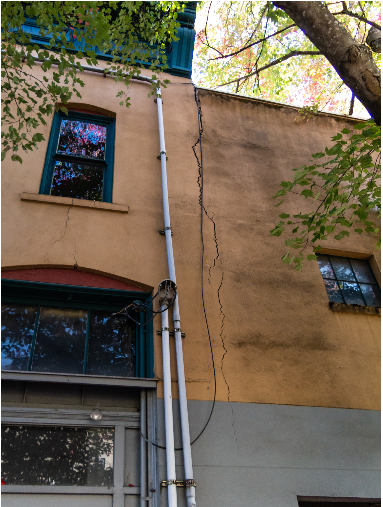
THE CRACK IN THE WEST WALL
