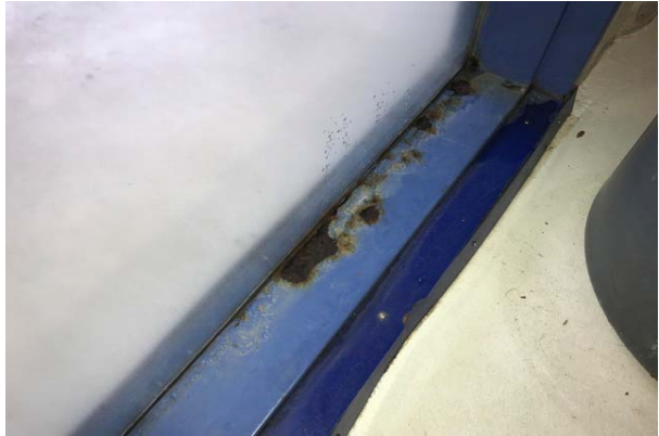
#20 DAMAGED WINDOW FRAME
