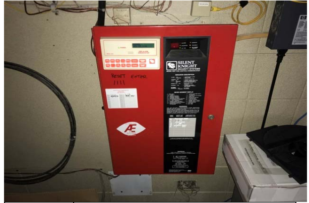
#50 FIRE ALARM PANEL
