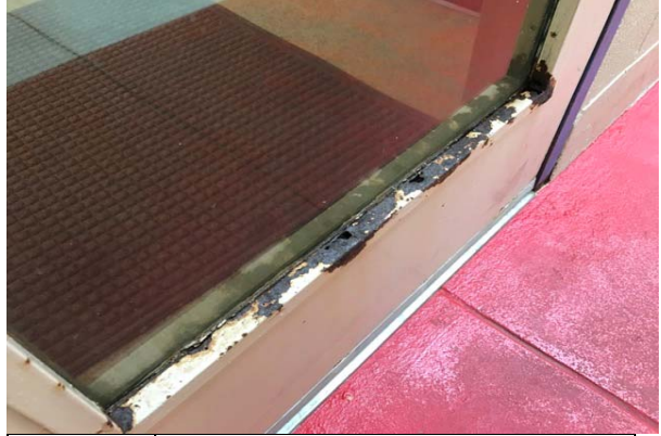
#38 INTERIOR DOOR, CORRODED
