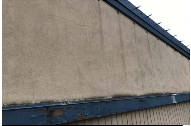
#14 DAMAGED STUCCO WALL ASSEMBLY AND TRIM
