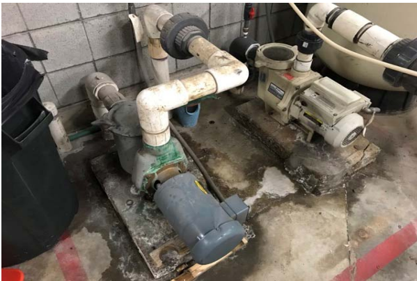
#53 POOL PUMP, SPA
