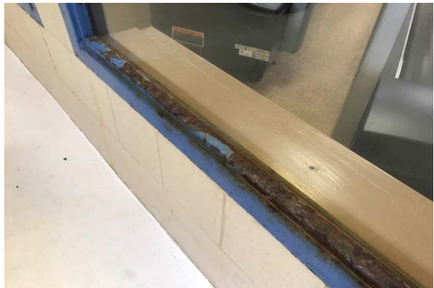
#36 DAMAGED INTERIOR WINDOWS
