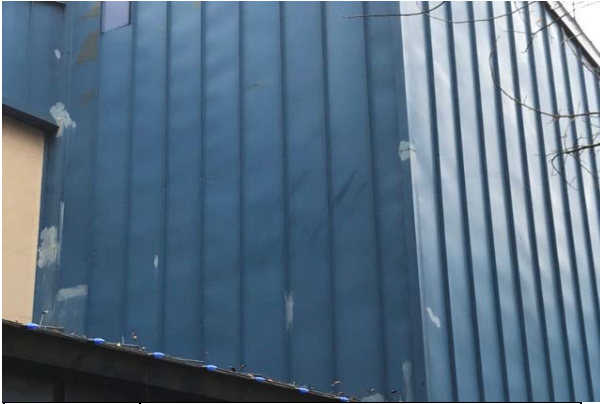
#13 DAMAGED METAL WALL PANELS
