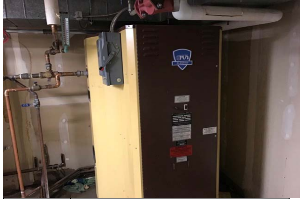
#38 FAILED DOMESTIC WATER HEATER
