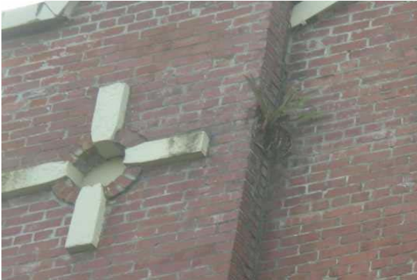
#13 DAMAGED MASONRY GROUT
