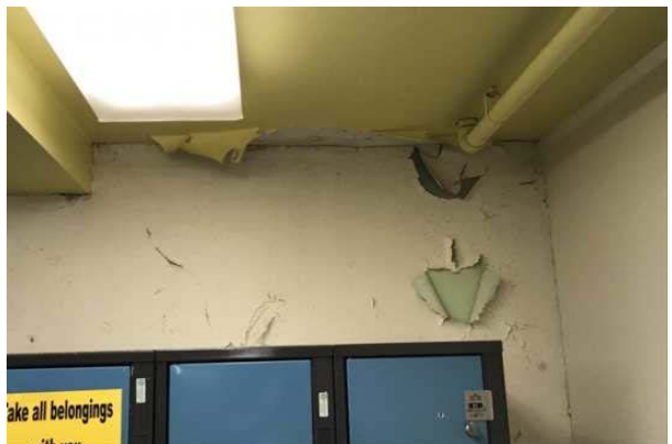
#18 WATER LEAK IN MEN'S LOCKER ROOM
