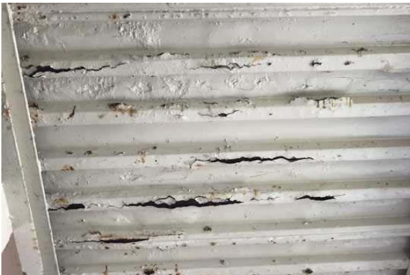
#23 FAILED STAIR LANDING
