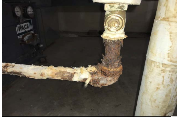
#32 HVAC SYSTEM HYDRONIC PIPING
