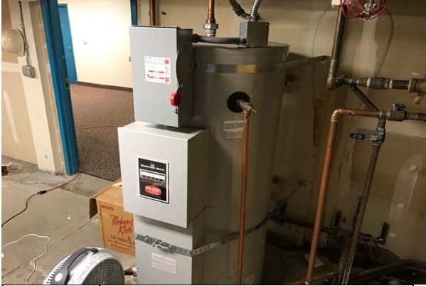
#37 DOMESTIC WATER HEATER
