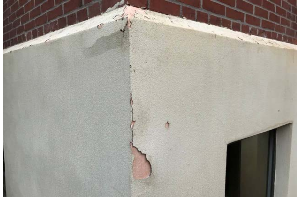
#14 DAMAGED STUCCO TEXTURE
