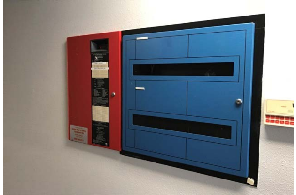
#34 FIRE ALARM CONTROL PANEL
