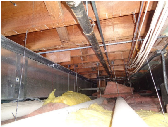
#15 ABOVE CEILING SPACE WITH UNBRACED PIPING AT BOTTOM
