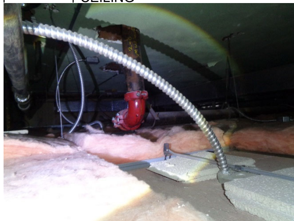
#18 BRACED FIRE SUPPRESSION PIPING
