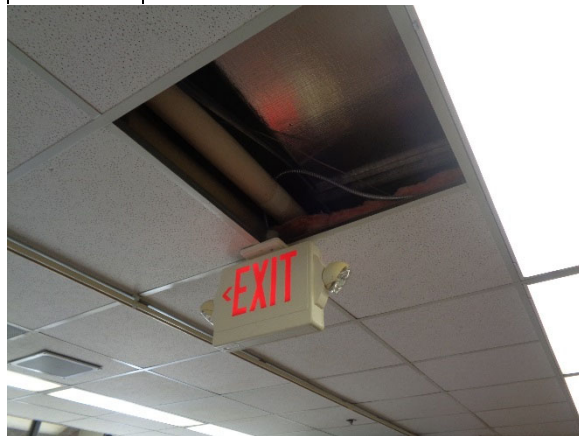
#16 EMERGENCY EXIT LIGHTING SUPPORTED BY SUSPENDED CEILING
