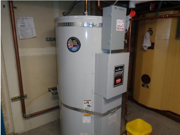
#13 RESTRAINED WATER HEATER
