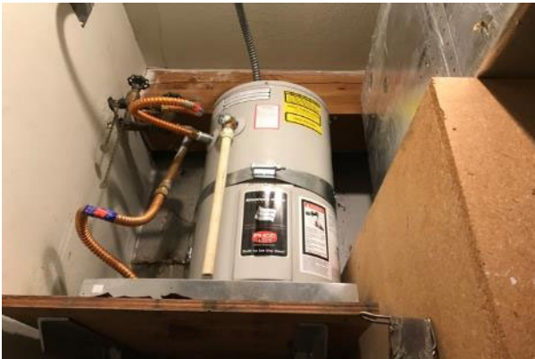
#45 WATER HEATER, ELECTRIC
