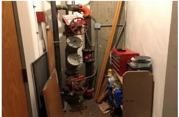
#16 FIRE SUPPRESSION BACKFLOW PREVENTER
