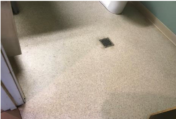
#69 INTERIOR FLOOR FINISH, VINYL SHEETING
