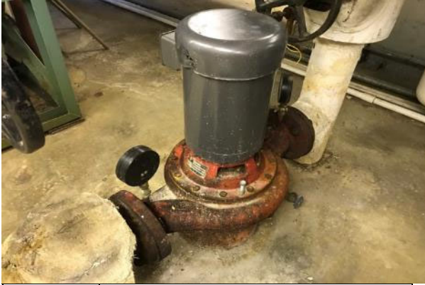
#49 CHILLED WATER AND CONDENSER WATER PUMPS
