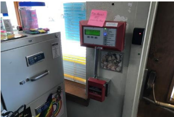
#63 ANNUNCIATOR ALARM PANEL
