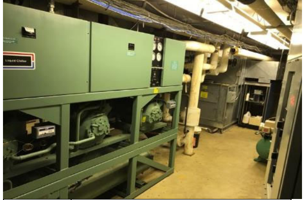
#20 LIBRARY MECHANICAL ROOM
