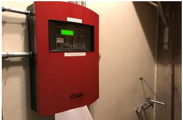
#60 FIRE ALARM CONTROL PANEL
