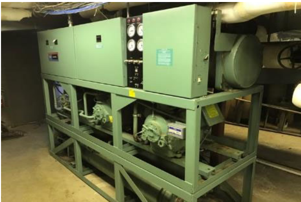
#47 WATER COOLED CHILLER
