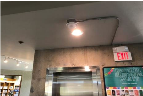
#15 FIRE ALARM SYSTEM
