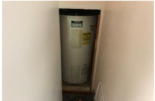
#46 WATER HEATER, ELECTRIC
