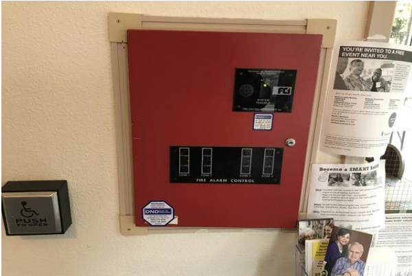
#61 FIRE ALARM CONTROL PANEL
