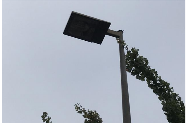
#14 POLE LIGHT, EXTERIOR
