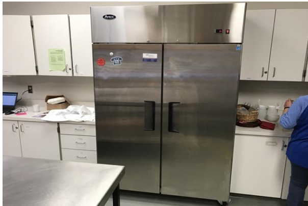
#70 COMMERCIAL KITCHEN, EQUIPMENT
