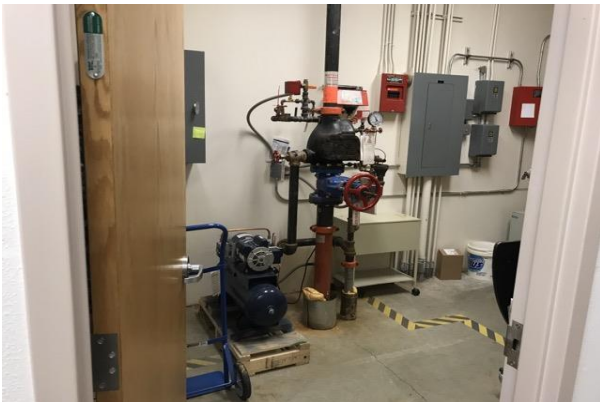
#65 SPRINKLER SYSTEM, DRY PIPE
