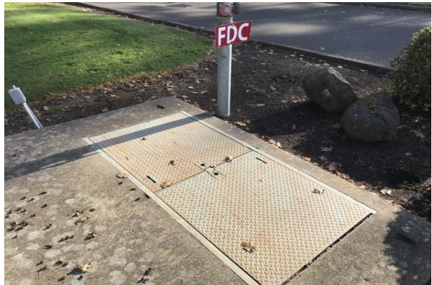
#64 FIRE MAIN LINE WITH BACKFLOW AND SIAMESE CONNECTIONS
