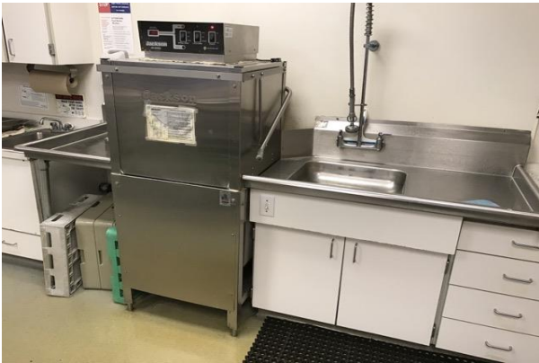
#69 COMMERCIAL KITCHEN, EQUIPMENT
