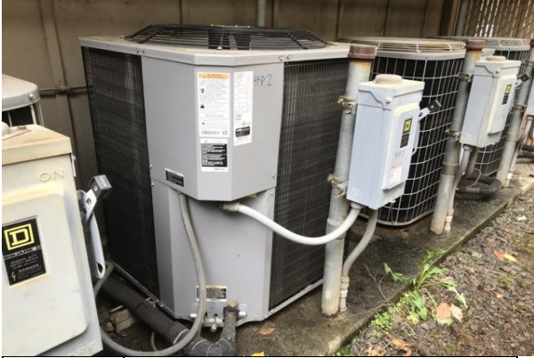
#43 CONDENSING UNIT/HEAT PUMP, SPLIT SYSTEMS
