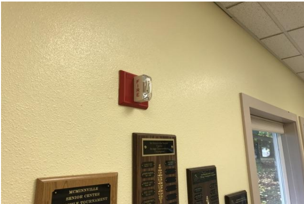
#63 FIRE ALARM STROBE
