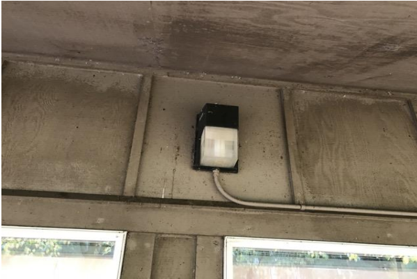
#13 COMPACT FLUORESCENT LIGHTING FIXTURE
