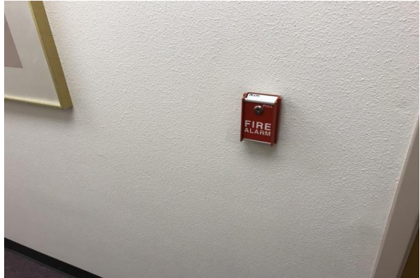
#62 FIRE ALARM PULL STATION
