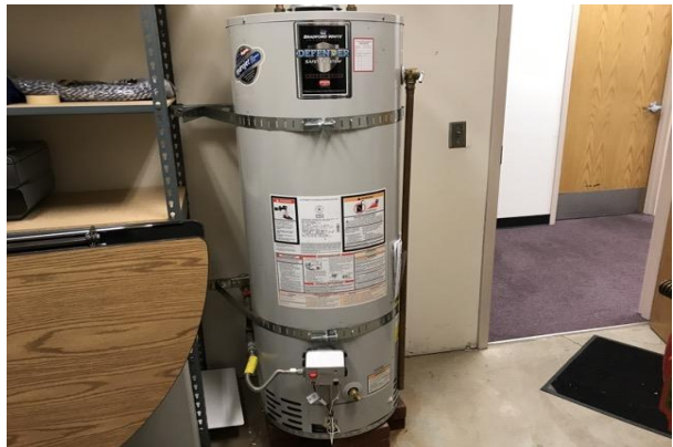
#48 WATER HEATER, GAS
