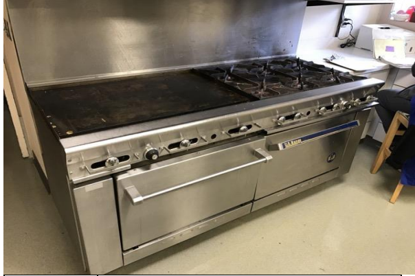
#68 COMMERCIAL KITCHEN, EQUIPMENT
