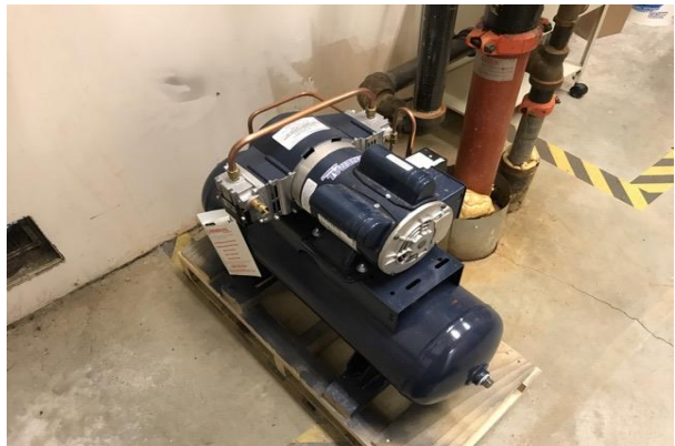
#66 DRY PIPE AIR COMPRESSOR
