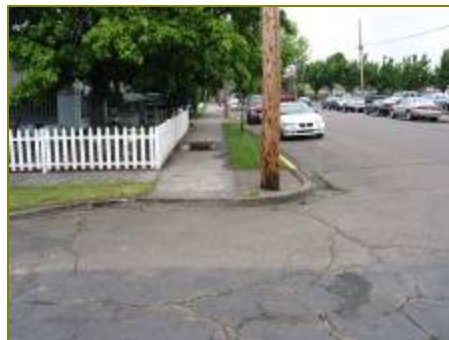
Missing Curb Ramp on 5 th Street
