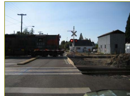
Missing Sidewalk at 5 th Street
