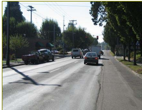
Rough Pavement on Adams Street
