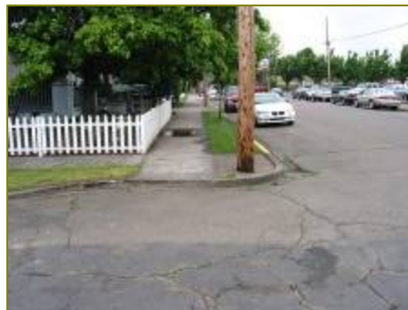
Missing Curb Ramp on 5 th Street
