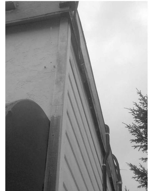
Existing SE corner, note lap siding on east wall of existing wood-framed addition.
