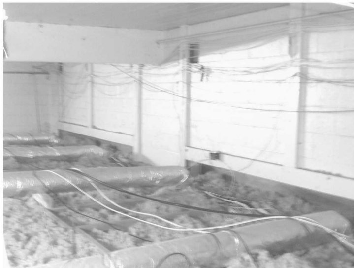
Attic - south wall. Note GLB bears on CMU, between 2 original openings of overhead doors. Note roof decking above, below is ceiling framing with batt insulation and HVAC ducts.
