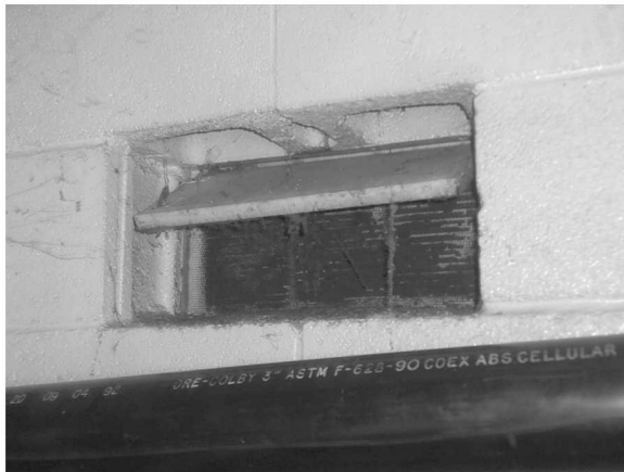
Existing north exterior CMU wall, attic vent in CMU gap. Note CMU above has no grout. Vents are typically dirty.
