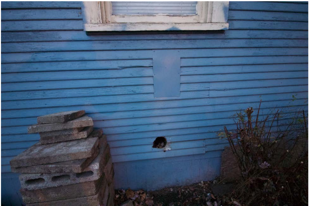
Large hole through house at East wall
