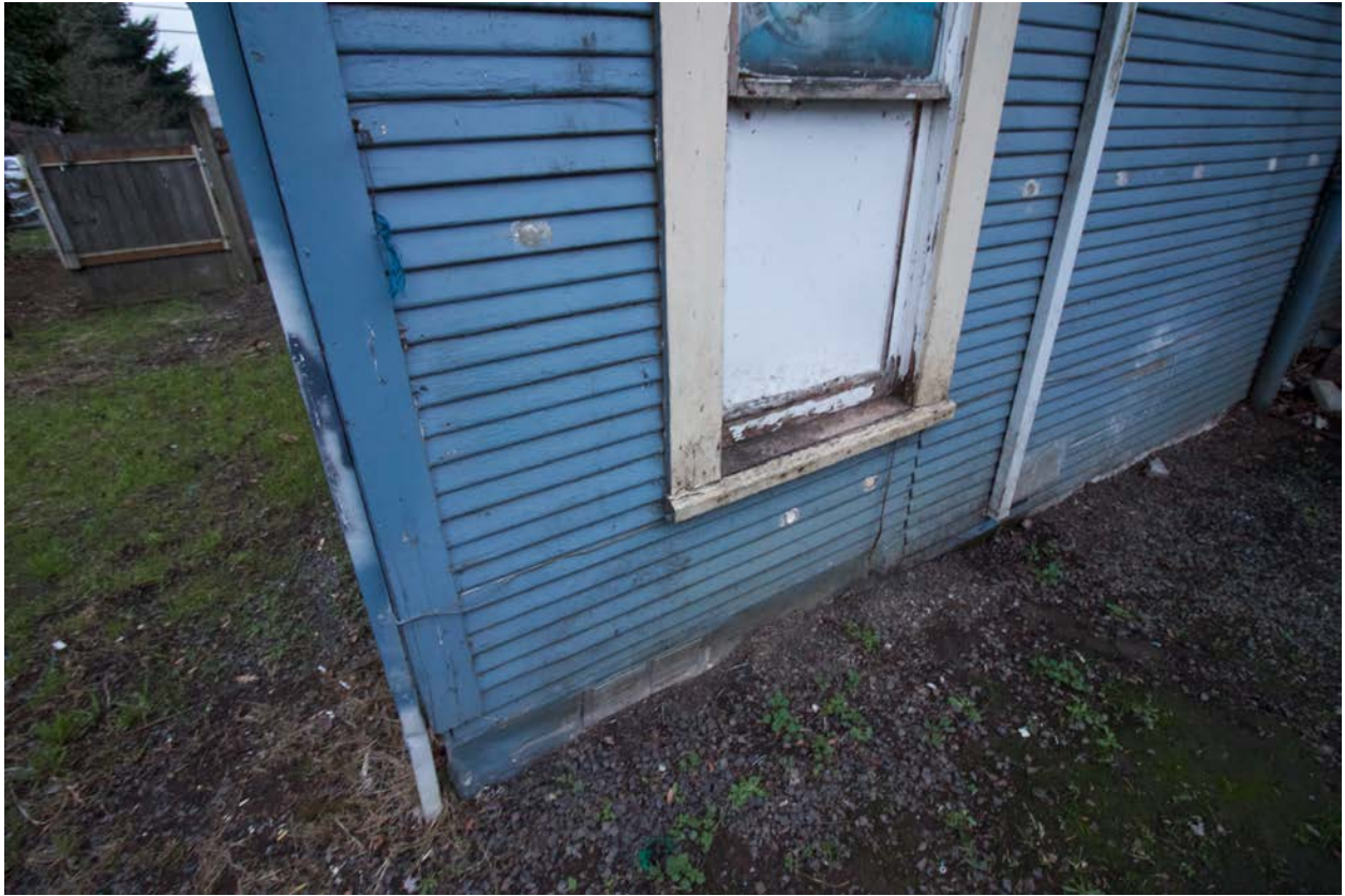
Window deterioration, missing glass, siding offset, untreated insulation holes
