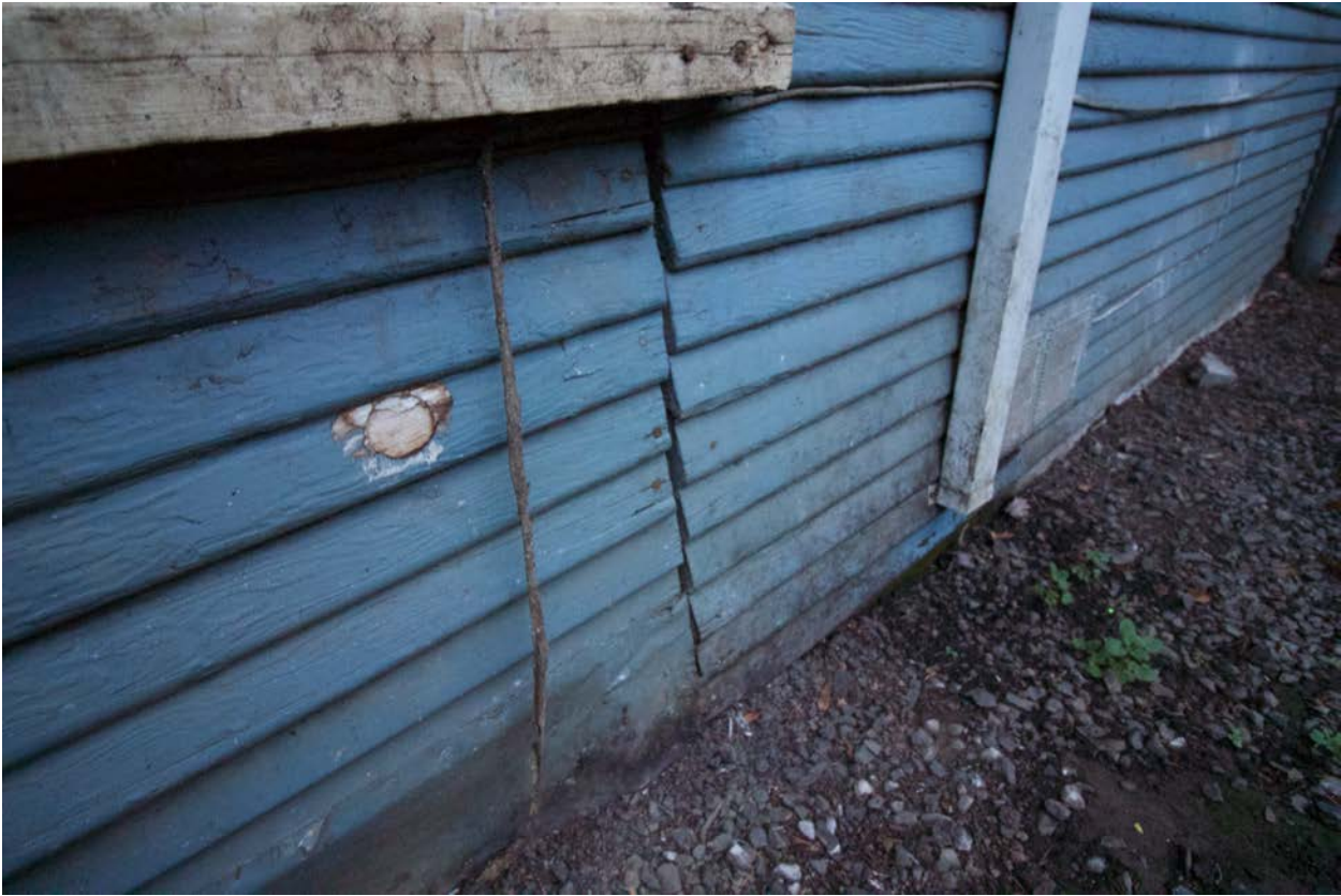
Close-up at exposed butt joint and misaligned siding
