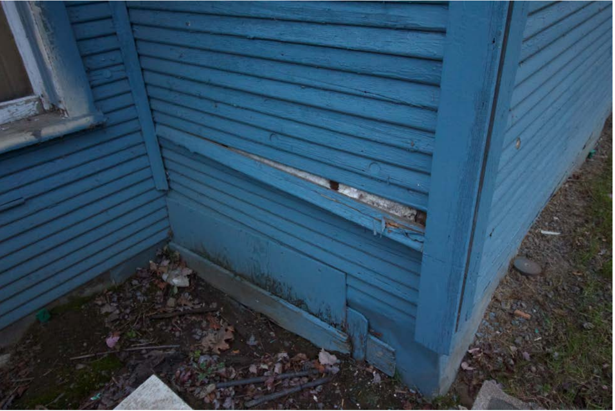
Siding falling off
