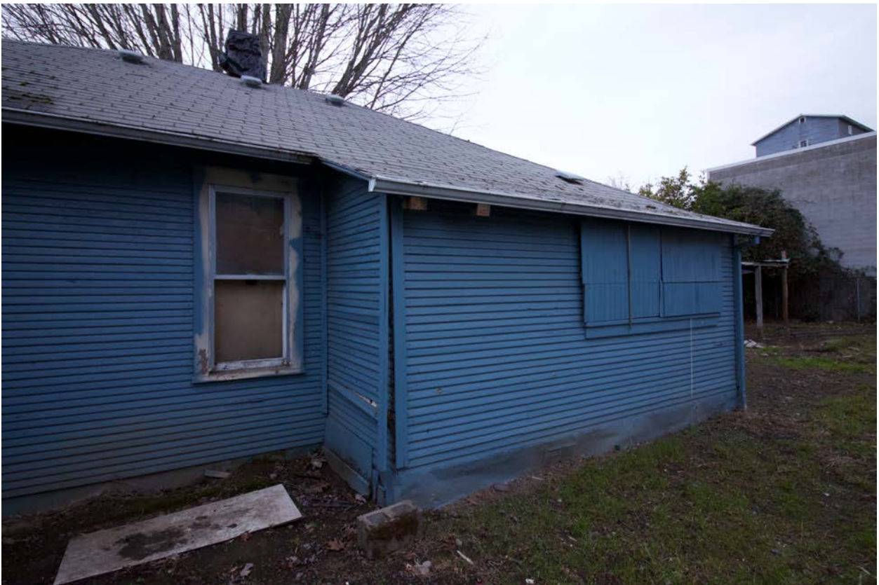
East side, no foundation, siding bowing out, boarded windows
