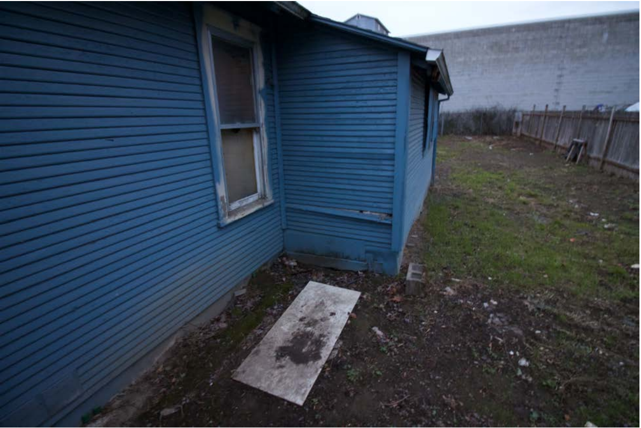
Siding falling off
