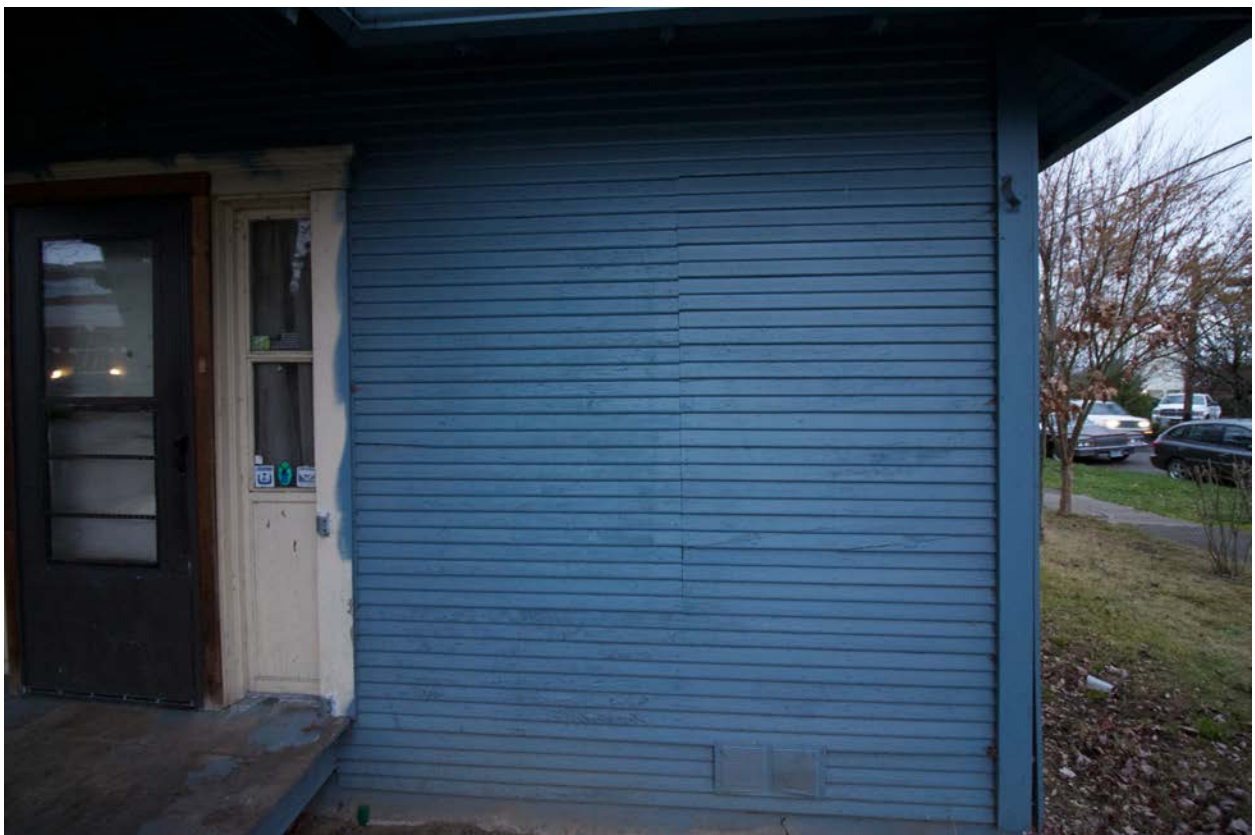
Butt joint and misaligned siding at East wall
