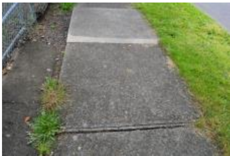
Sidewalk damage and trip hazards
