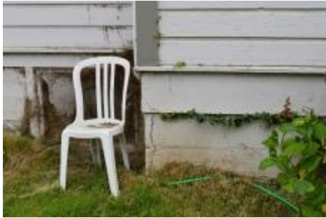
Foundation cracks and separation from the building
