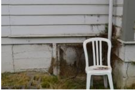
Foundation cracks and separation from the building
