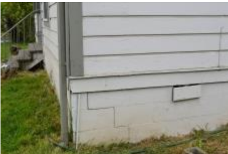
Foundation cracks and separation from the building
