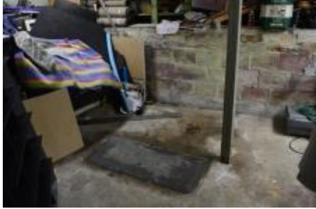
Basement flood damage, pooling moisture
