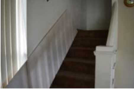
Inside stairwell, Not up to code. Too narrow and steep
