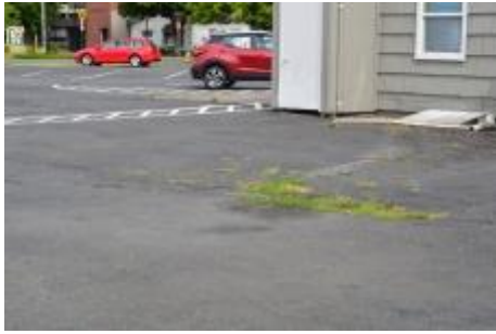
Parking lot damage
