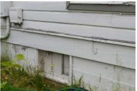
Dry rot to exterior, holes in foundation
