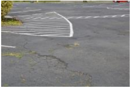
Parking lot damage and trip hazard
