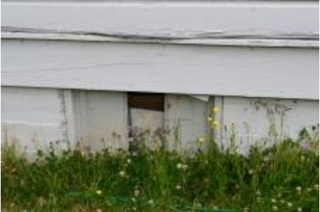
Dry rot to exterior, holes in foundation
