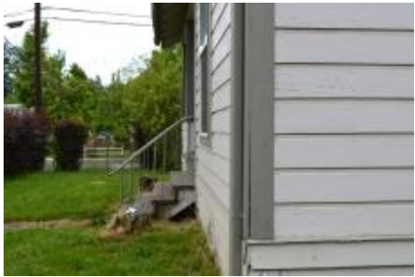
Exterior stairwell, Dry rot and broken rails
