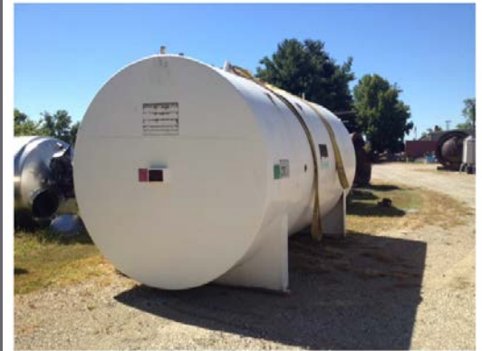
Photo No.2: This is a photo of a 12,000 gallon fuel tank.
