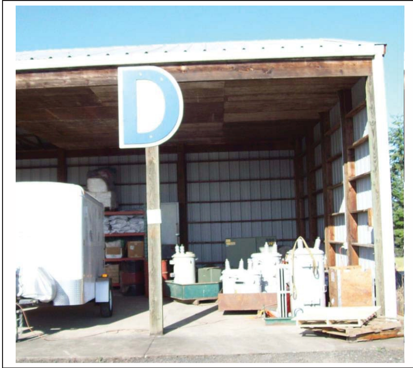
Containment Area in Pole Shed for Damaged Transformers Awaiting Pickup
