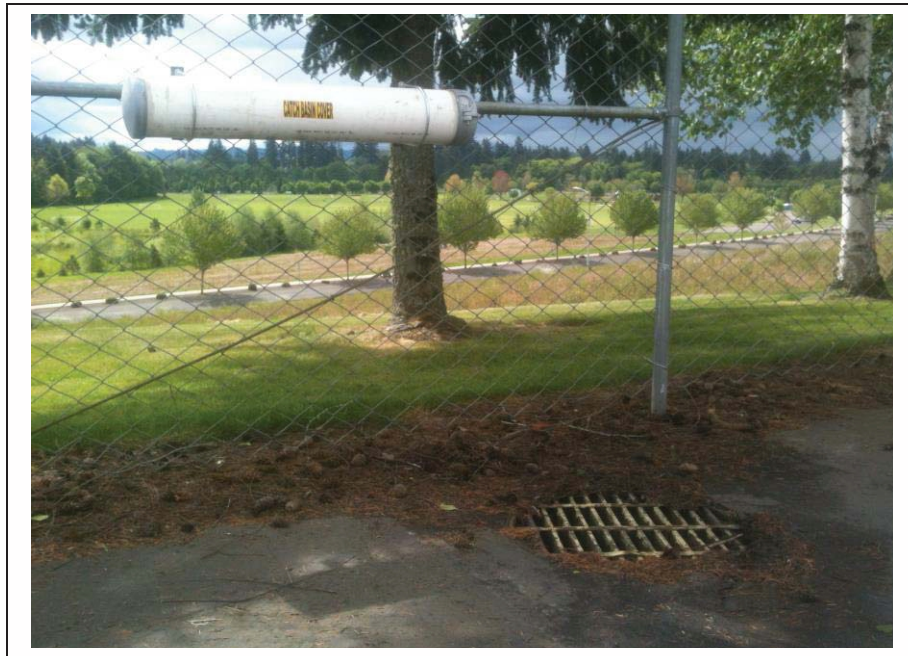
Catch Basin Cover near Catch Basin by Southern Fence
