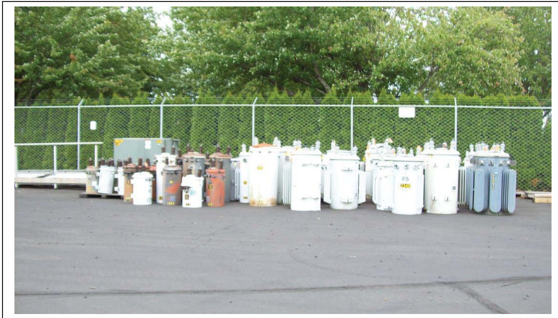
Transformer Disposal Storage Area
