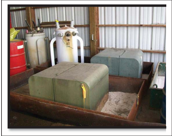
Damaged Transformers in Containment
