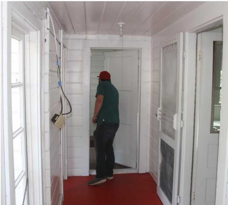
Figure 15: View from North within current porch structure of door to garage area (worker entering). This door to be replaced in new plan by an exterior door in essentially the same location.
