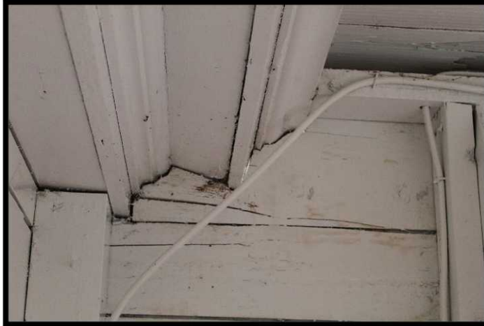
Figure 5: View from within porch addition structure. Note roofline (upper left) of main house preserved with notched interior wall to fit
