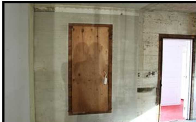
Figure 4: Boarded-up exterior window on East-facing interior wall discovered during demolition
