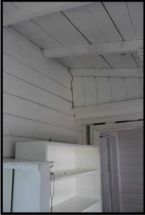
Figure 2: View from within porch addition. Note exterior siding (left) on interior wall
