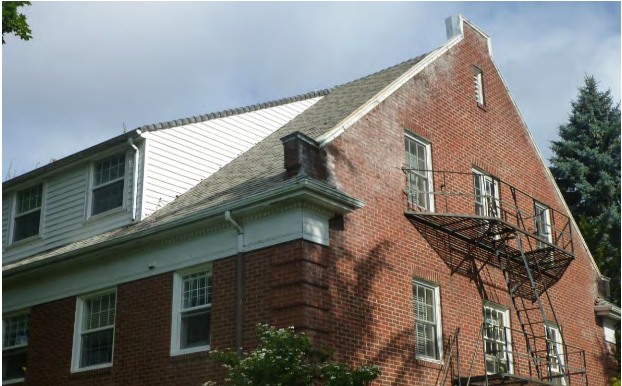
View of southeast building corner showing brick decay
