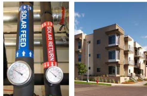
RECOMMENDED - solar hot water and sun shading which is incorporated into the architecture of the building.
