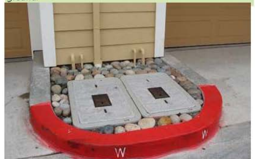
NOT RECOMMENDED - Meters and other utilities located within previously planned landscape areas due to conflicts with plan coordination.
