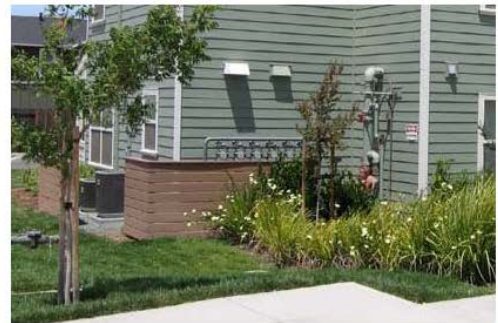
RECOMMENDED - Meters and other utilities should be screened with landscape or low walls when above ground.
