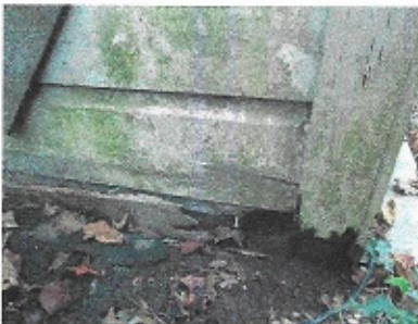
Extensive dry rot
