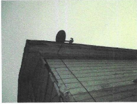
Extensive dry rot, no gutters
