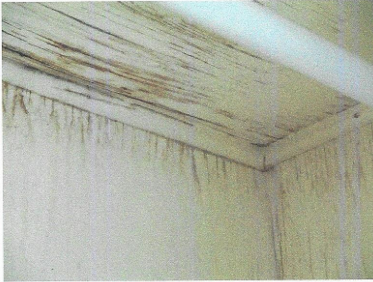
Interior extensive water damage, dry rot.
