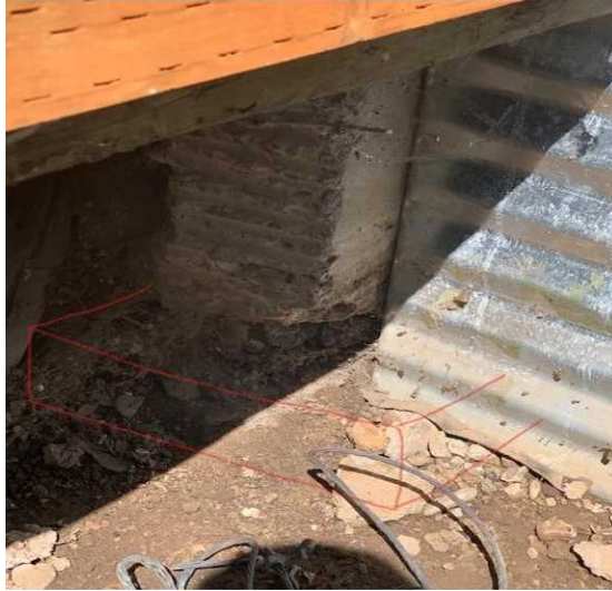
Image 8 College 423 No foundation footing (Similar to College 415)
