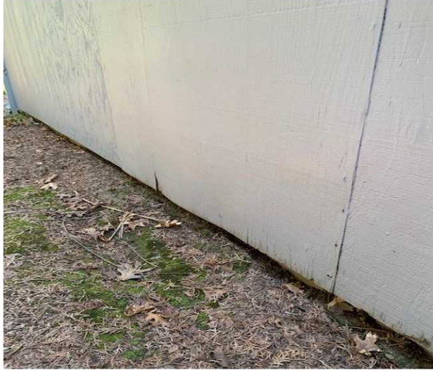
Image 6 College 415 Siding and sole plate dry rot.
