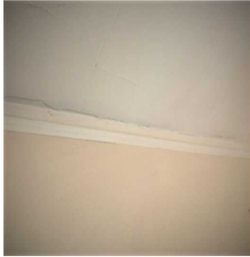
Image 10 College 423 Roof structure detaching from load bearing wall.
