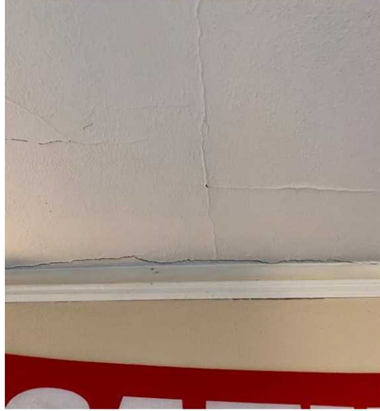
Image 12 College 415 Roof structure detaching from load bearing wall.
