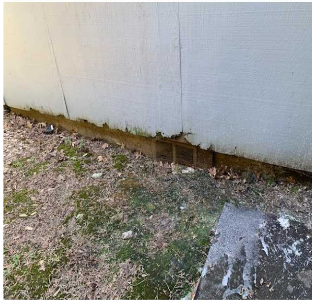
Image 7 College 415 Siding dry rot.
