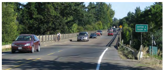
Limited Sidewalk Width on Yamhill River Bridge
