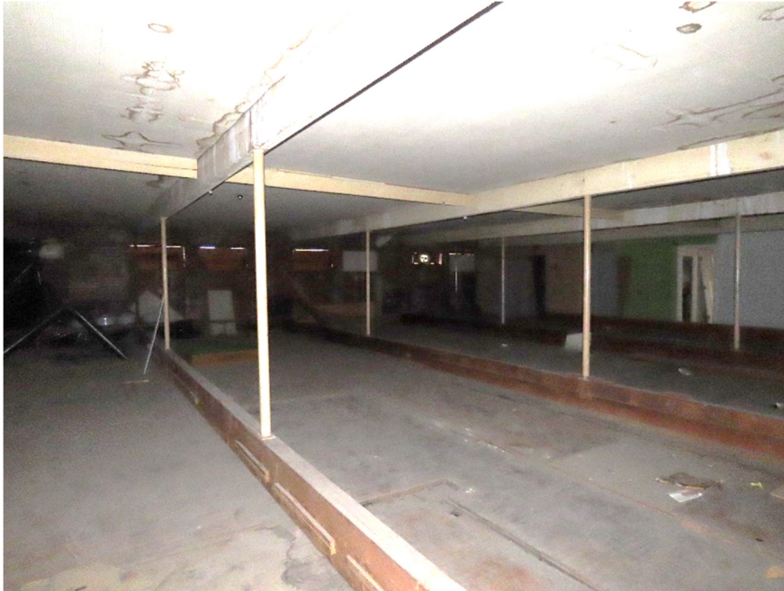
Photo 19. Round pipe columns at second floor with areas of removed partitions (ARG, October 2022).
