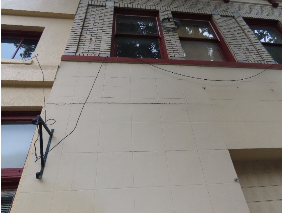
Photo 11. South elevation, crack at non-original stucco, original windows and masonry at second floor (ARG, October 2022).
