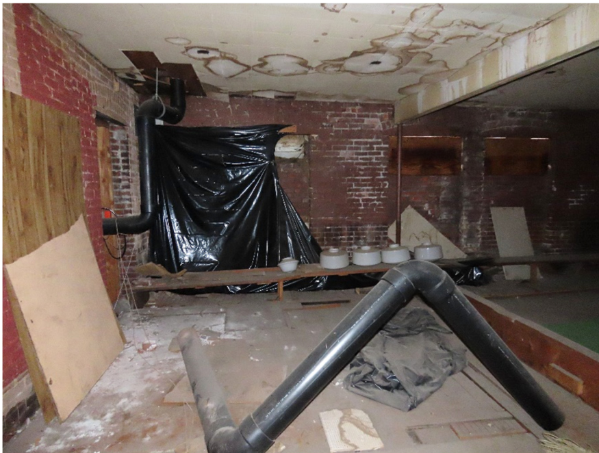
Photo 20. Second floor north wall with removed windows, damaged finishes below clogged drain (ARG, October 2022).
