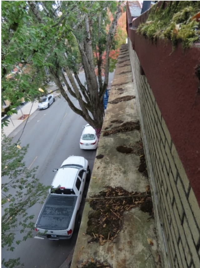
Photo 15. Top of cornice, with areas of biological growth (ARG, October 2022).
