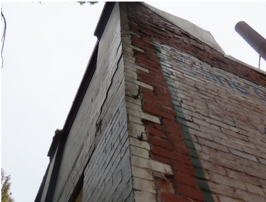
Photo 22. Southwest corner, note cracking and outward masonry displacement at attic story (ARG, October 2022).
