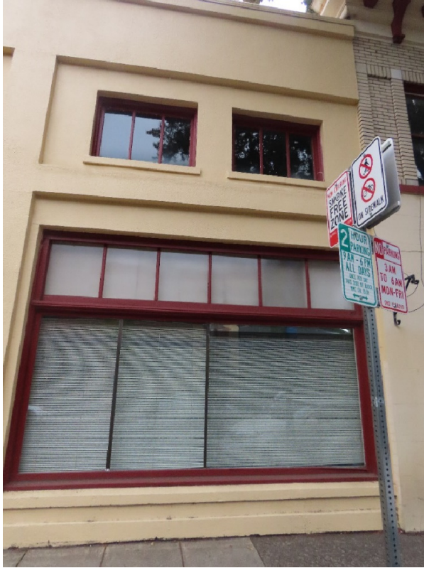
Photo 1. NE 3rd Street elevation: Original wood storefront window and transom, and second-floor windows; storefront has been modified with addition of metal mullions (ARG, October 2022).
