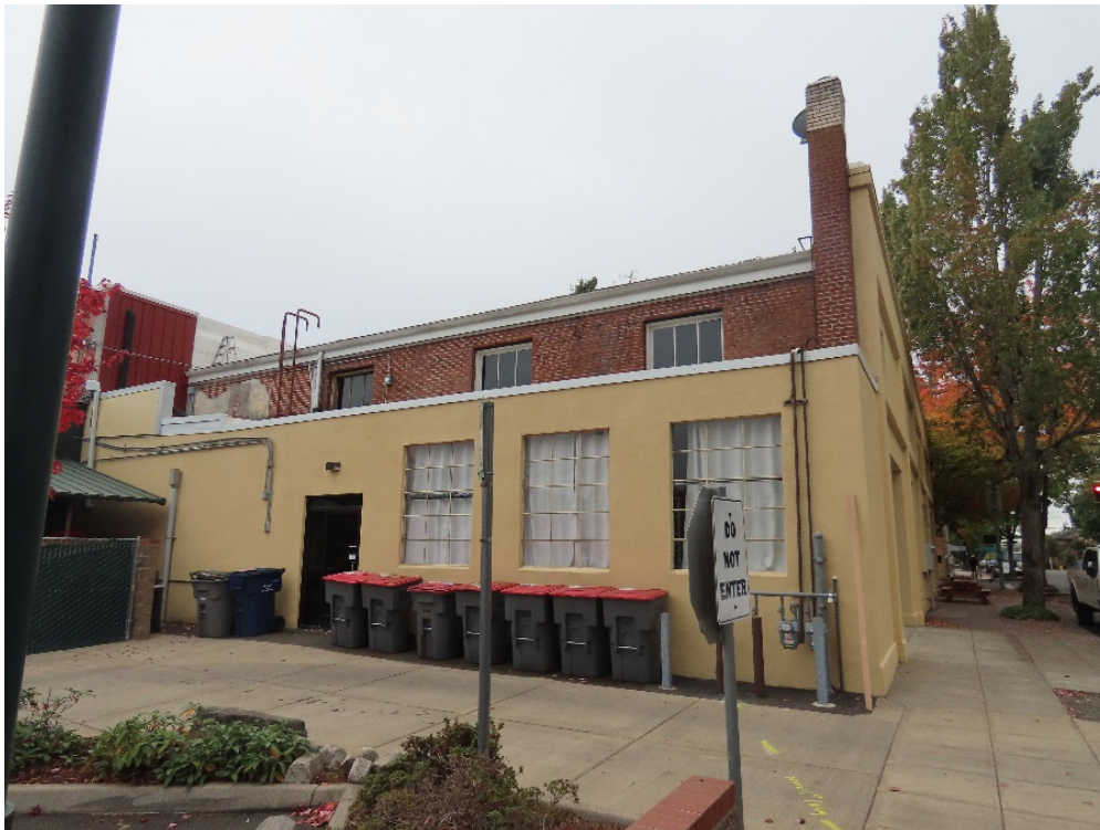
Photo 6. One-story north bay, rear elevation, showing original second floor windows, And steel windows at ground floor (ARG, October 2022).
