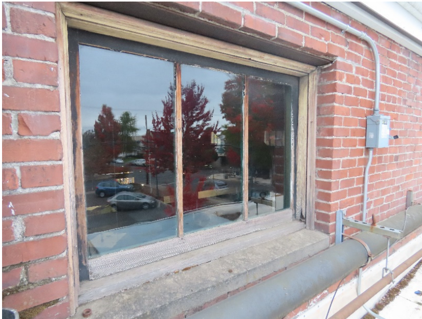
Photo 4. Second floor window, north (rear) elevation, with nearly complete loss of paint, and putty bead loss. Note wood deterioration at right lower jamb (ARG, October 2022).
