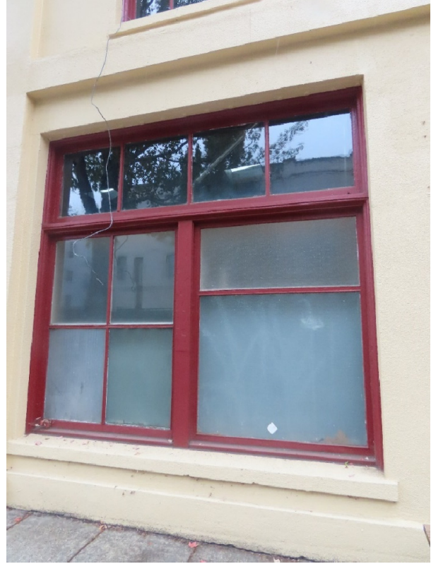
Photo 2. NE Ford Street elevation: Original wood storefront window and transom; mis-matching translucent glass types. Storefront muntins may have been reconfigured (ARG, October 2022).
