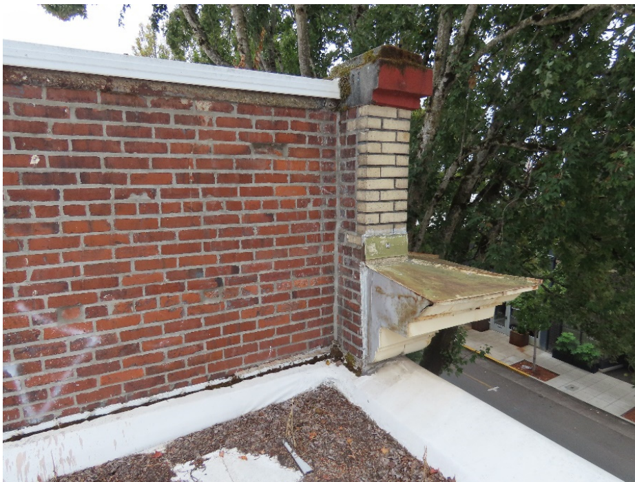
Photo 10. Parapet and top of metal entablature exhibiting minor corrosion (ARG, October 2022).
