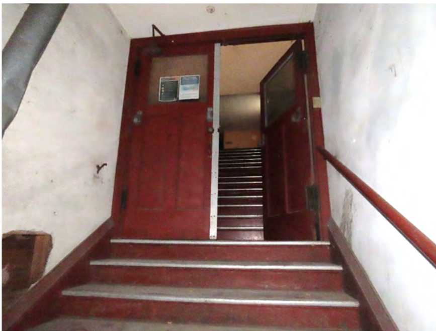
Photo 18. Original pair of doors at SE stair to second floor (ARG, October 2022).
