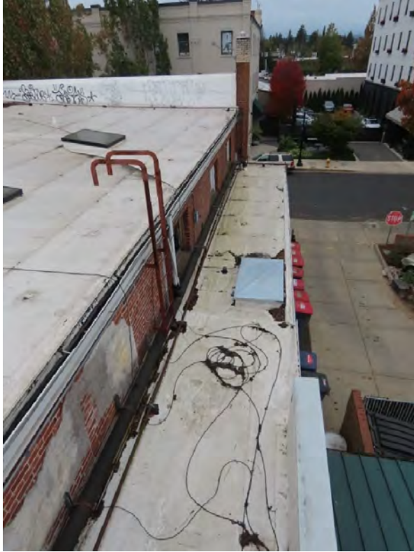
Photo 5. Replacement roofing; main roof at left, one-story north bay at right (ARG, October 2022).
