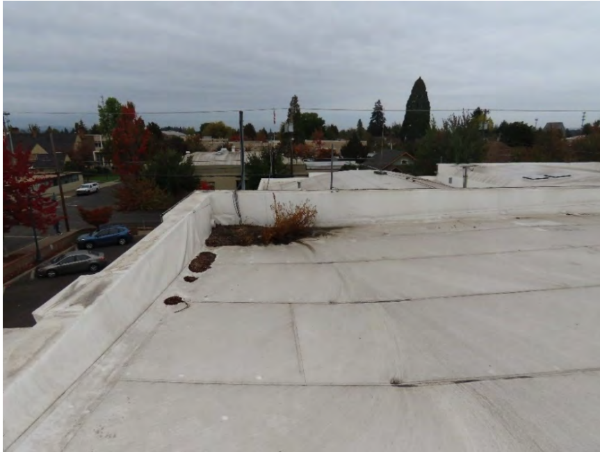
Photo 17. Roof looking north; note debris at location of roof drain (ARG, October 2022).
