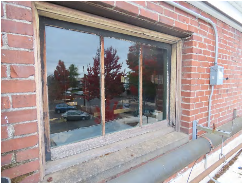
Photo 4. Second floor window, north (rear) elevation, with nearly complete loss of paint, and putty bead loss. Note wood deterioration at right lower jamb (ARG, October 2022).
