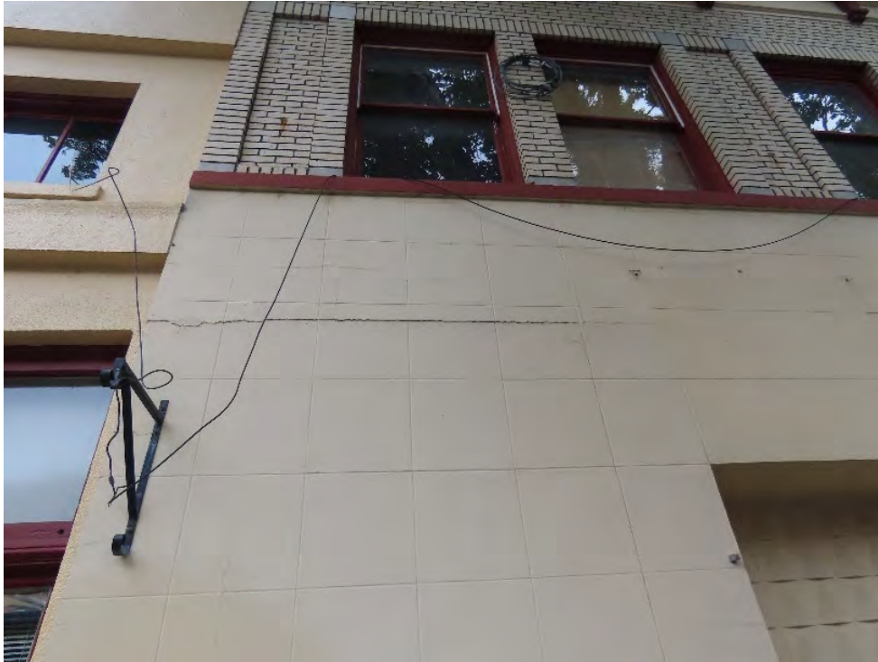
Photo 11. South elevation, crack at non-original stucco, original windows and masonry at second floor (ARG, October 2022).
