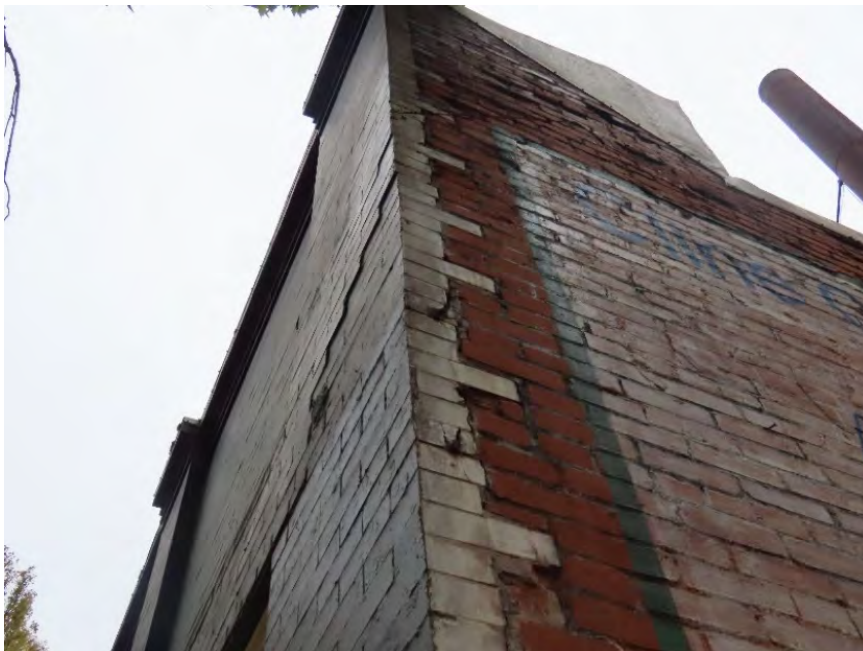
Photo 22. Southwest corner, note cracking and outward masonry displacement at attic story (ARG, October 2022).
