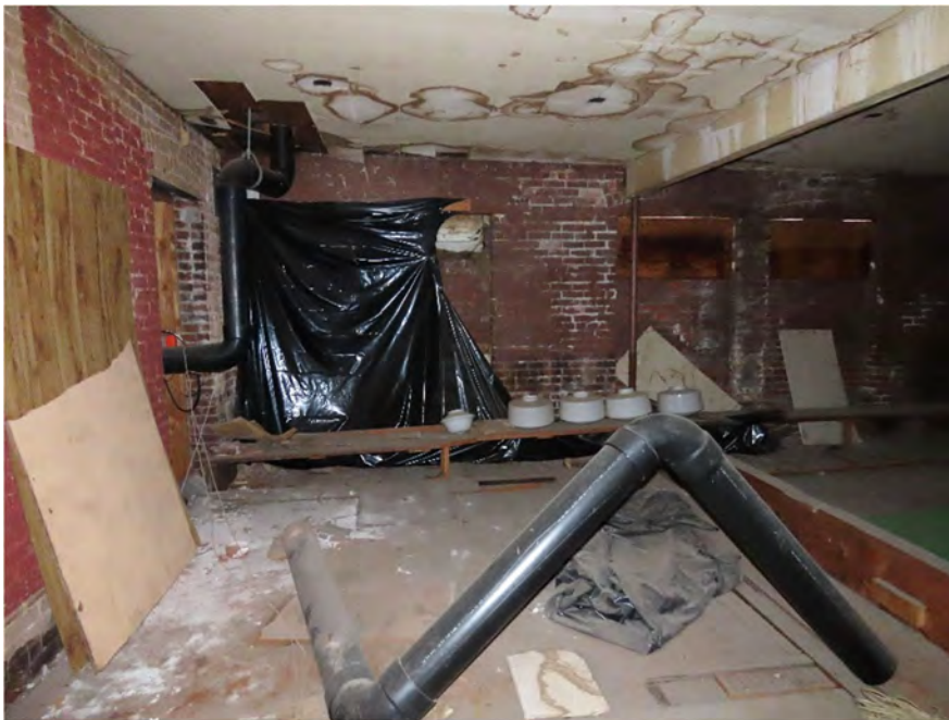
Photo 20. Second floor north wall with removed windows, damaged finishes below clogged drain (ARG, October 2022).
