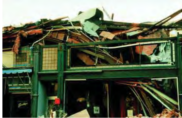
■ Figure 5. Destruction of a historic building.
