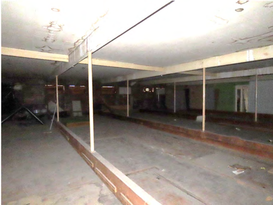
Photo 19. Round pipe columns at second floor with areas of removed partitions (ARG, October 2022).
