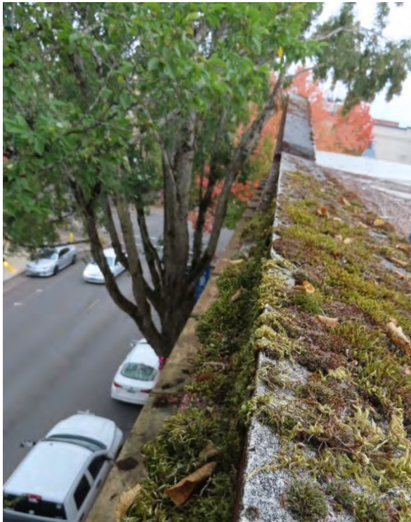
Photo 14. Top of coping with significant biological growth (ARG, October 2022).
