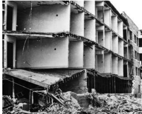
■ Figure 14. Heavily damaged Hotel Californian, 1925 Santa Barbara, California earthquake. —NISEE, U.C. Berkeley
