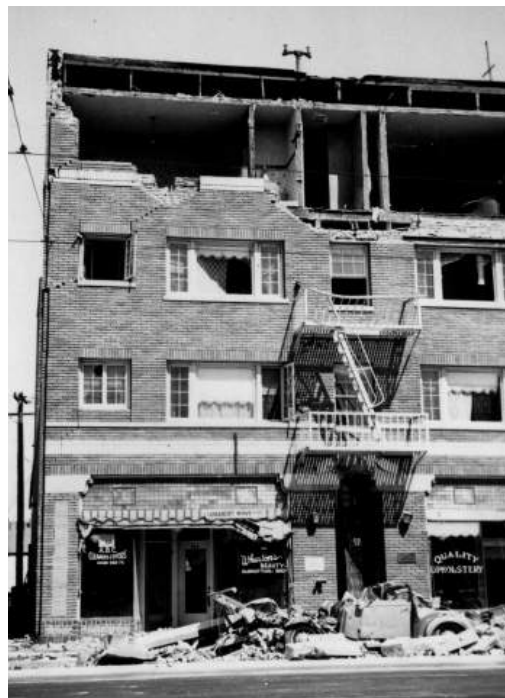
■ Figure 15. URM building damage, 1933 Long Beach, California earthquake. —Los Angeles County Public Library
