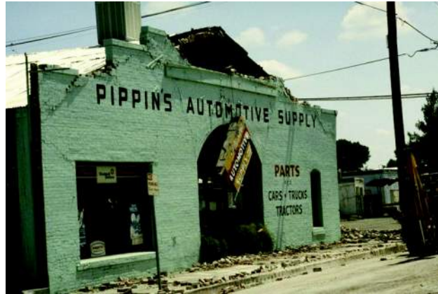
■ Figure 16. URM building with end-wall failure, 1983 Coalinga, California earthquake. Robert Reitherman —NISEE, U.C. Berkeley
