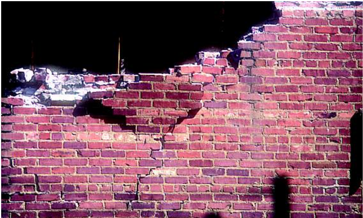
■ Figure 6. Damaged URM wall in a red-tagged building, fated to be torn down or to undergo a multi-year closure for repairs and upgrading.
