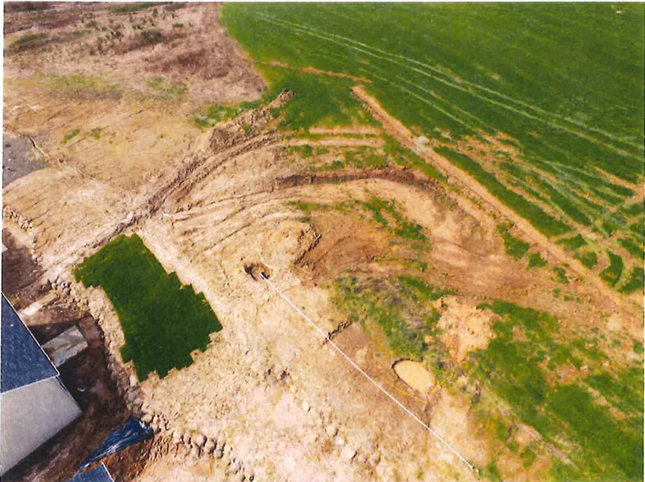
Existing, Recently Active Landslide – View to the West March 17, 2016
