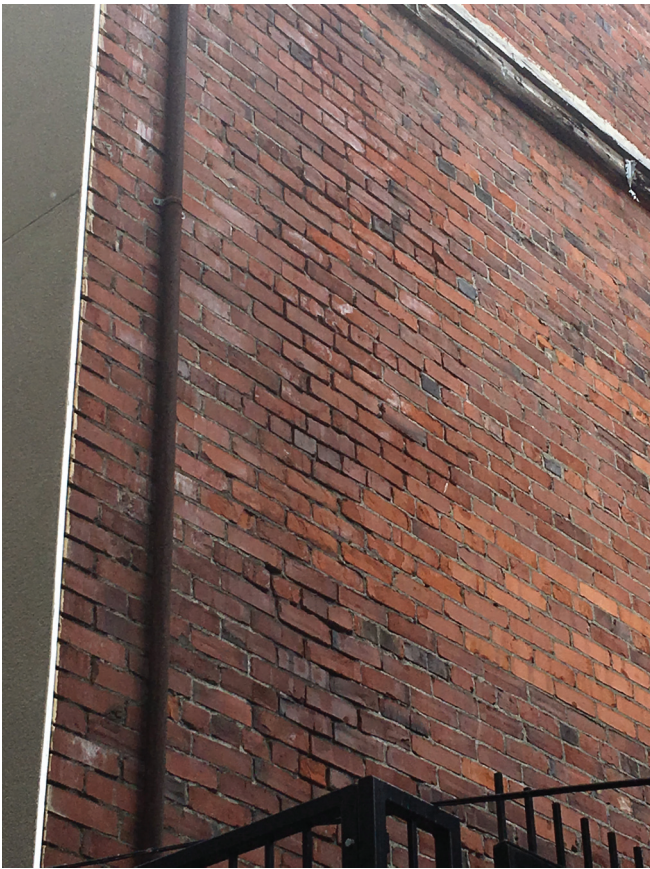
DETERIORATED RED BRICK AT EAST FACADE
