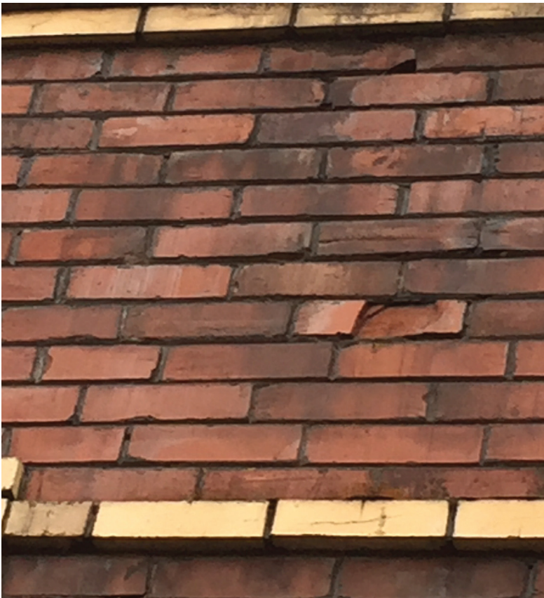
SPALLING RED BRICK AT NORTH FACADE
