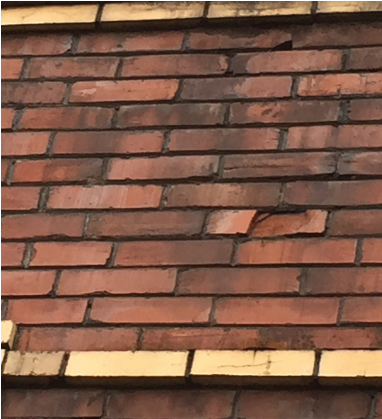
SPALLING RED BRICK AT NORTH FACADE
