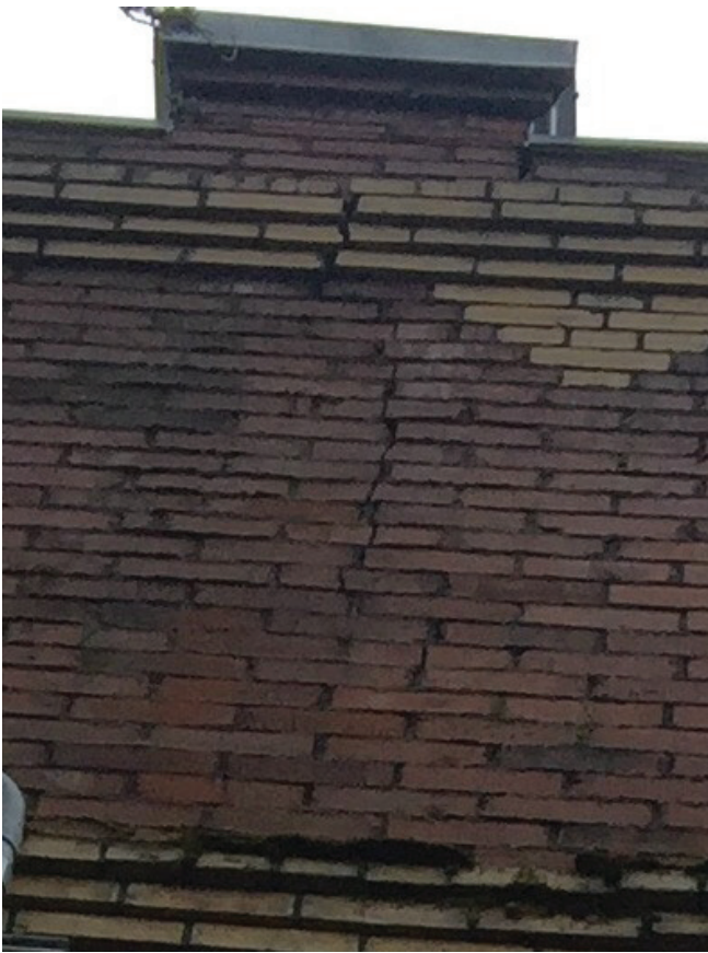
SPALLING RED BRICK AND CRACKING AT NORTH FACADE
