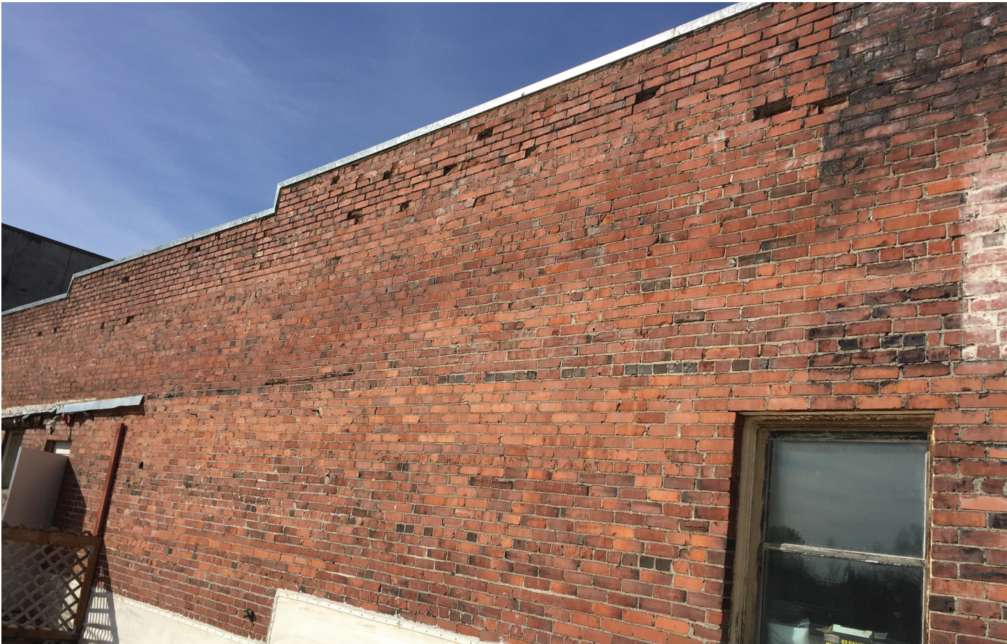
EAST FACADE, SHOWING MISSING AND DAMAGED BRICK
