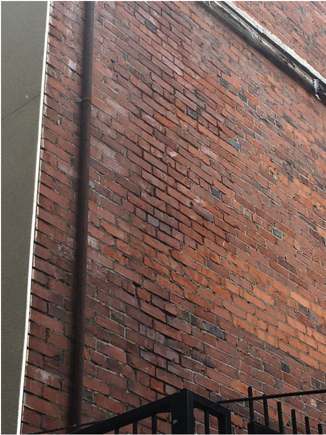
DETERIORATED RED BRICK AT EAST FACADE
