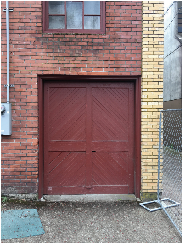
VERTICAL LIFT RAMP DOOR
