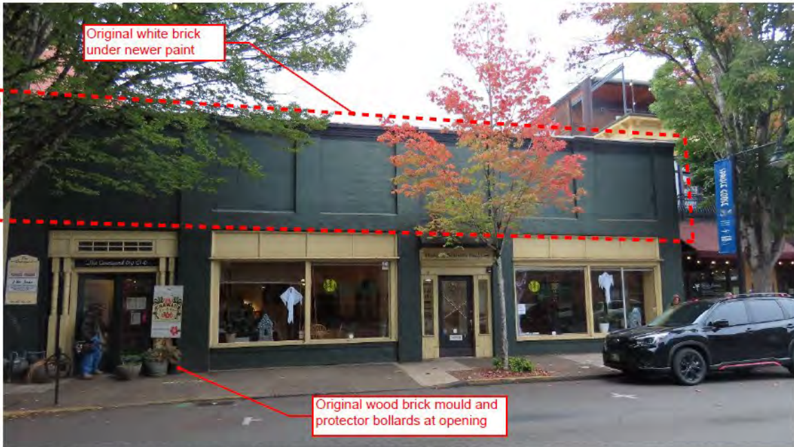
Current view of 619 NE 3rd Street (ARG, October 2022). Paired doors with wood trim elements have been inserted into the westernmost bay, while the formerly double-wide opening has been replaced with a storefront window matching the window in the easternmost bays.
