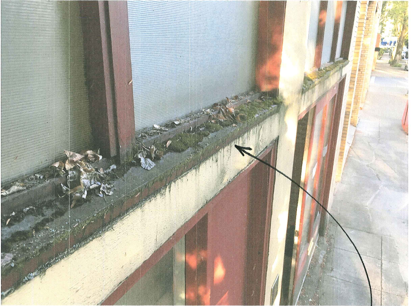
TRANSOM WINDOW SILL CONDITION
