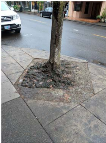
Construction likely to significantly disturb or destroy already-fragile roots
